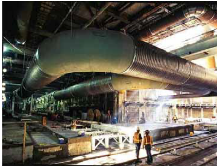
Figure 4-19: Underground Ventilation Ducts
