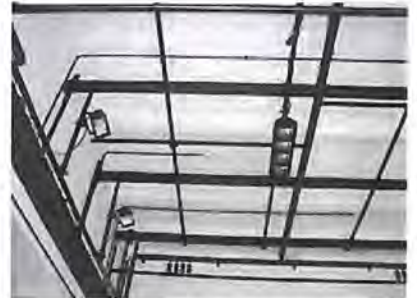
Ceiling with light fixtures for stage in the Festsaal
