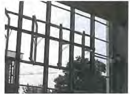
Mechanically opened windows
