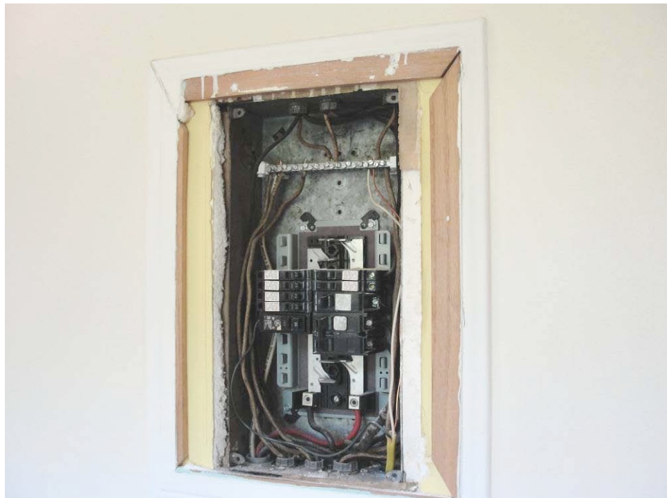
PHOTO: This is the panel in the laundry.
