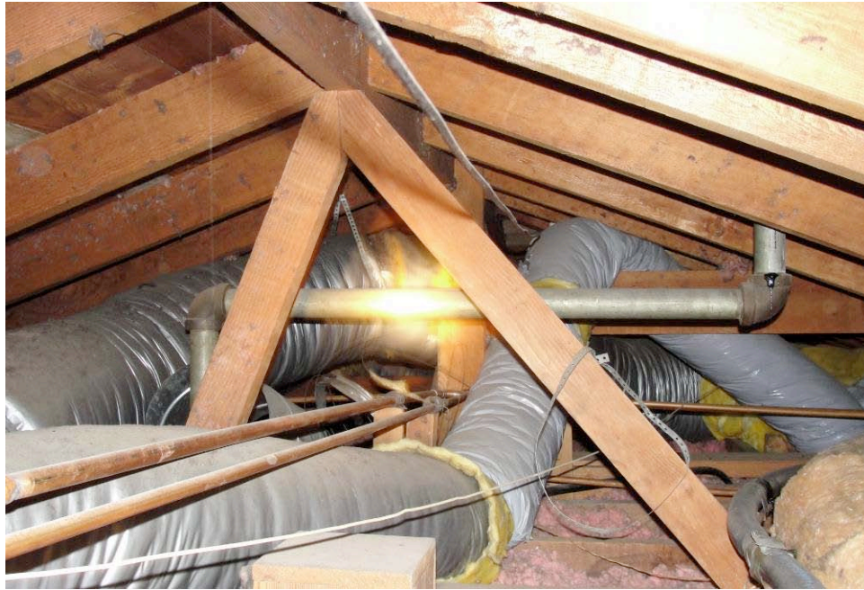
PHOTO: A view of the upper attic, looking north from the hall access hatch.
