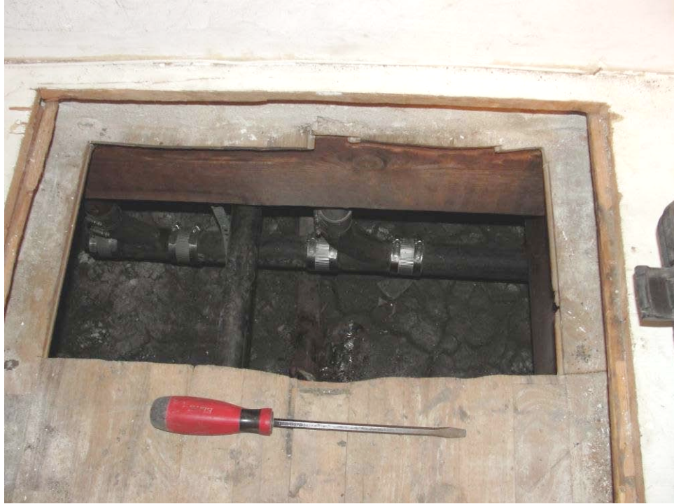
PHOTO: This is the hatch in the east maid's room. The screwdriver was placed to provide scale.
