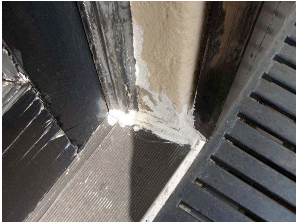
PHOTO: The joints at the threshold of the doors at the master bedroom have been caulked.
