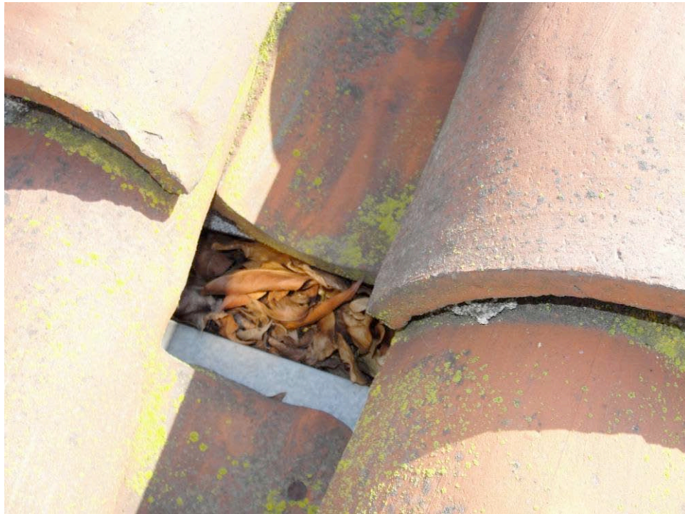
PHOTO: The blind gutters are clogged at some locations.
