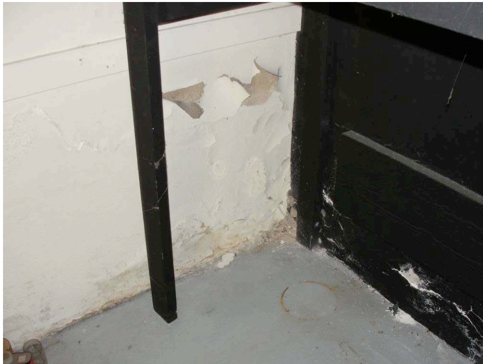
PHOTO: The south east corner of the garage is water damaged.
