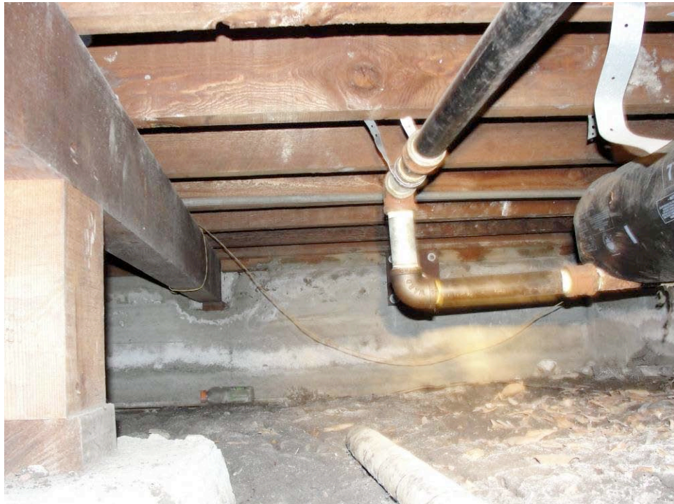
PHOTO: This photo was taken "blind" from the hatch in the bedroom. It is looking east. Note the good condition of the concrete foundation wall. Also note the presence of the foundation anchor (directly behind the gas line in the center of the photo.)
