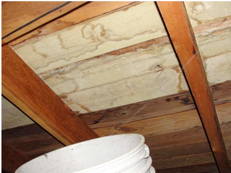
PHOTO: This water stain and the bucket below it were found in the lower attic, above the laundry.
