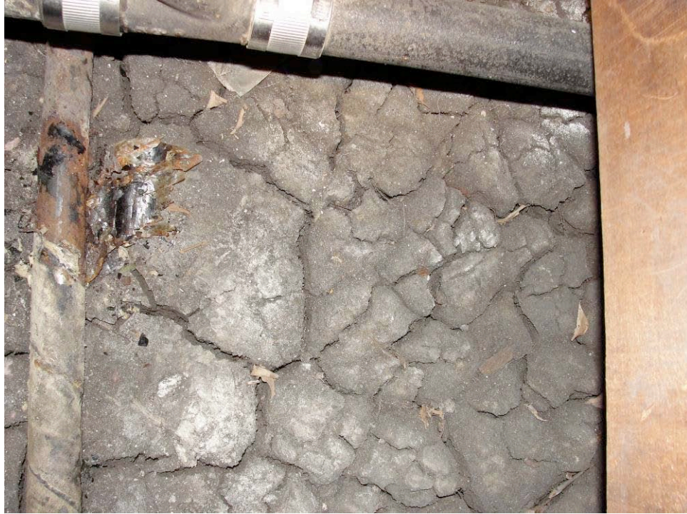
PHOTO: The cracked earth is an indication of expansive soils and past excessive moisture. Also note the damaged “field wrap” on the gas line in the left of the photo. See PLUMBING SYSTEMS notes below.
