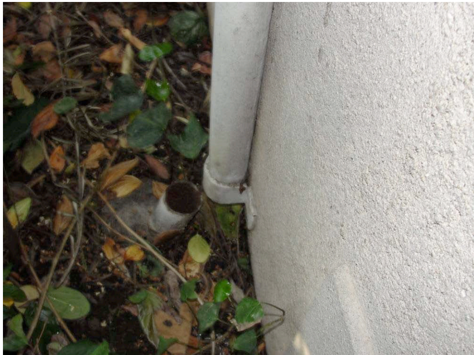
PHOTO: This separated drain will contribute to the adverse site drainage conditions.
