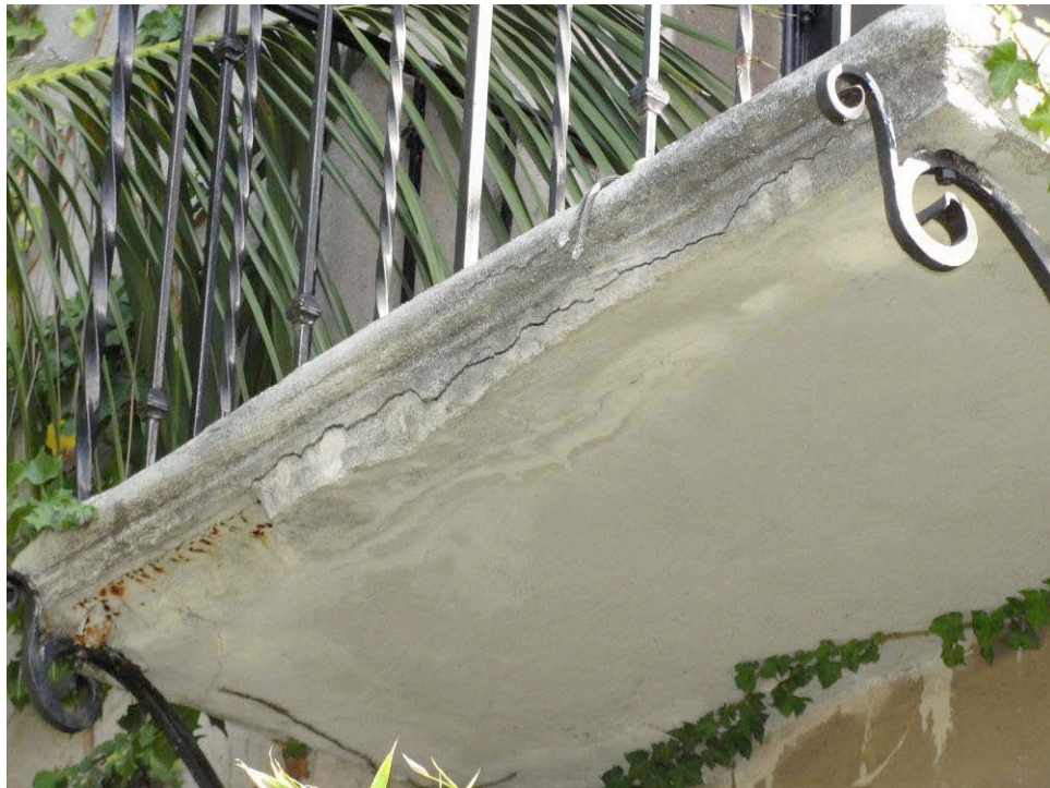
PHOTO: The concrete balcony at the north west bedroom is damaged.
