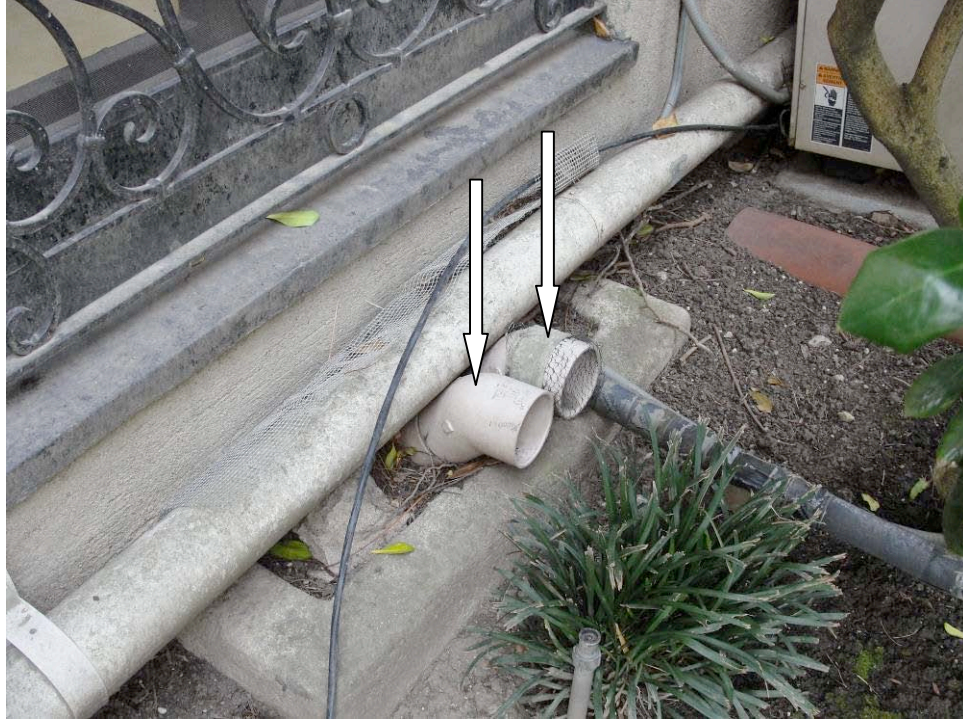
PHOTO: The exhaust and intake of the downstairs furnace are close.
