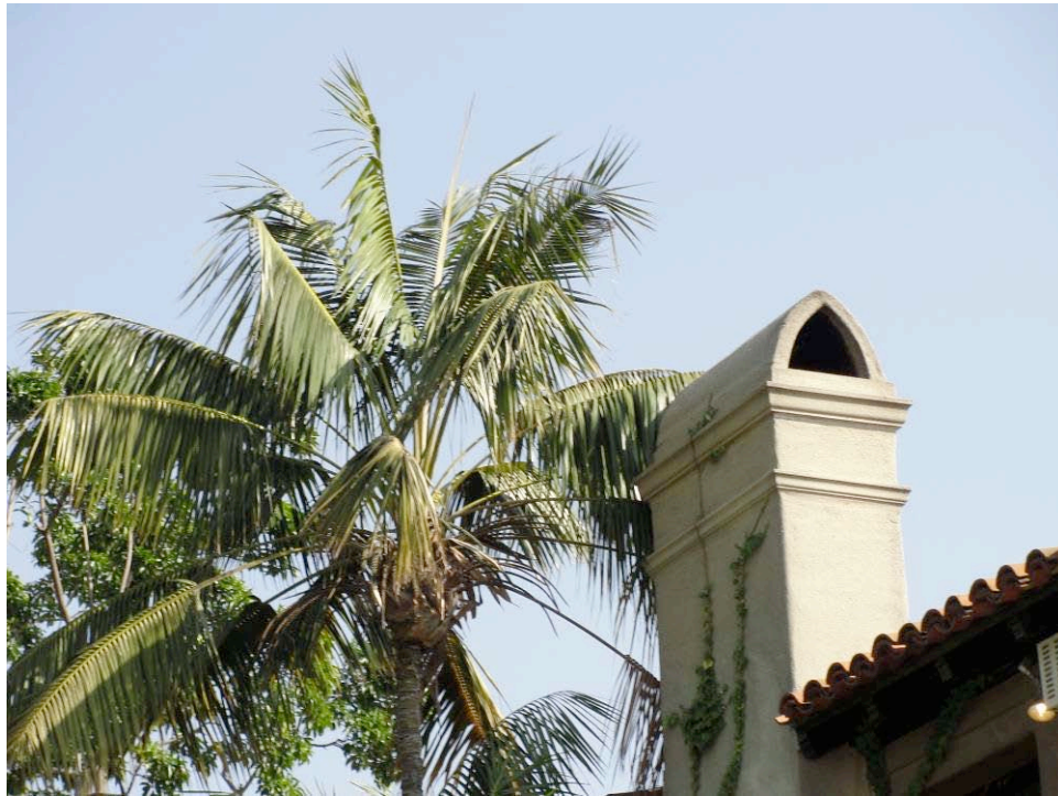
PHOTO: A palm tree is too close to the top of the den fireplace chimney.
