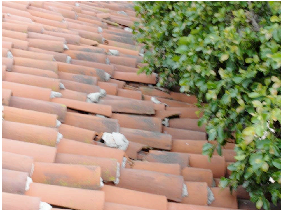
PHOTO: This is the area on the east side of the lower roof. Note the many damaged tiles.
