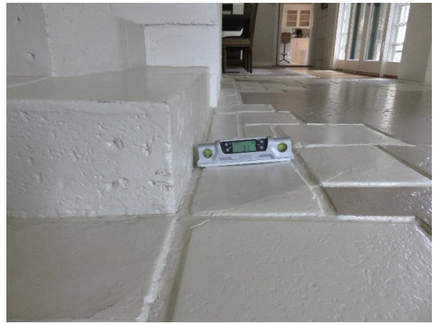
FIGURE 110. Uneven surface and bowing of the concrete entry slab.
