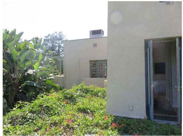
FIGURE 57. Mechanical equipment visible on the second floor roof.
