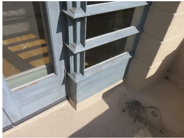
FIGURE 119. Peeling paint and wood deterioration at original west balcony doors.
