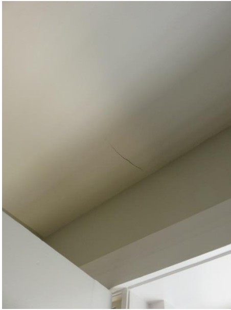
FIGURE 104. Cracked plaster above the west door in the northwest bedroom.
