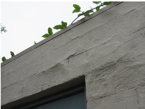
FIGURE 60. Cementitious parge coat surfacing at east elevation. Note delamination of surfacing and scoring of joint lines to match concrete block joints.
