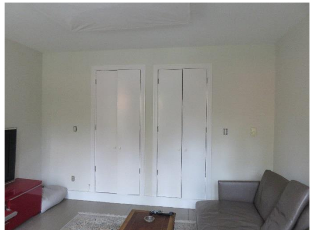
FIGURE 91. View of the west wall of the family room, which divides this space from the garage.
