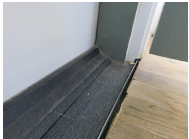
FIGURE 67. Gap between the floor boards and sill flashing on the east balcony doors.
