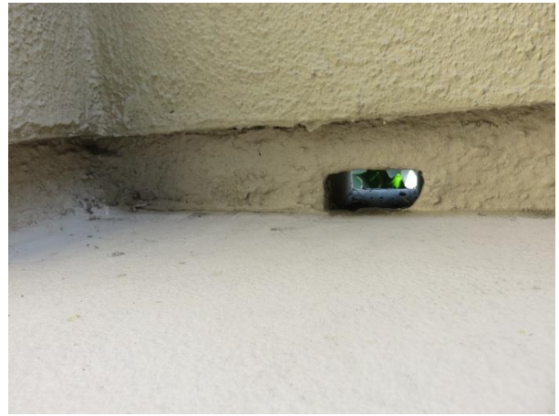
FIGURE 24. Scupper through the balcony wall.
