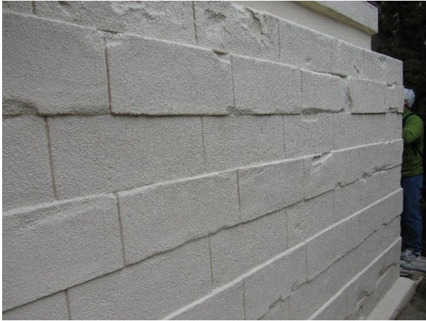
FIGURE 58. Spalls and surface scaling that has been covered with coating at the west elevation.
