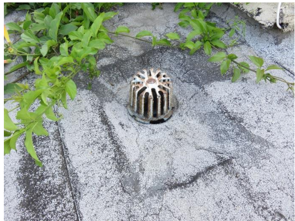
FIGURE 70. Deteriorated membrane around the roof drain.
