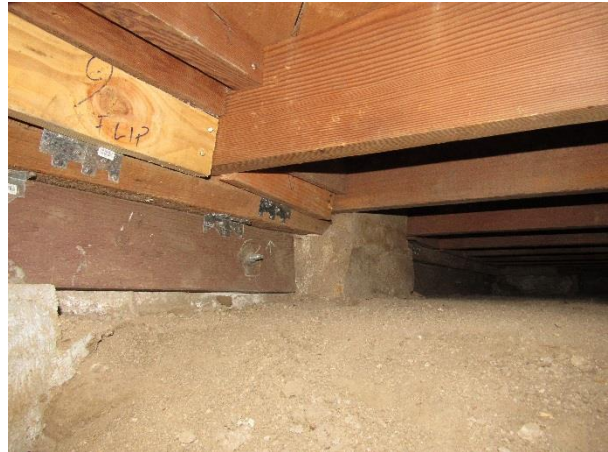
FIGURE 108. Strengthening measures at southeast crawlspace, including new plate bolted to foundation with new blocking and connections between joists and foundation and sill plate.
