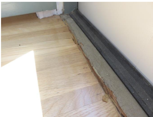
FIGURE 105. Cracked wood sill on the west door of the northwest bedroom.
