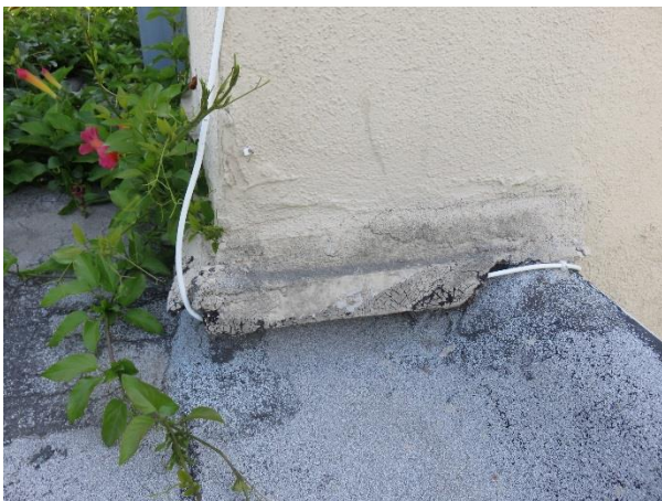
FIGURE 69. Deteriorated flashing at the roof to stucco-clad wall transition.
