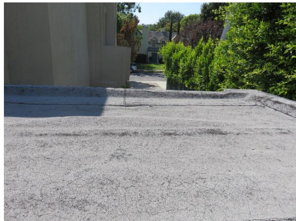
FIGURE 120. Area where the roof membrane is blistered and not bonded to the substrate.
