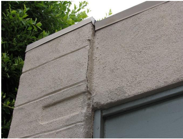
Figure 63. Cracking at a change of plane in the exterior wall.
