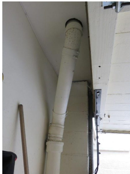
FIGURE 115. Cast iron roof drain pipe.
