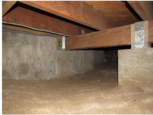
FIGURE 107. Typical wood framing, with wood beam framed into thickened concrete footing foundation (chimney location).
