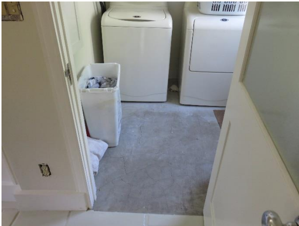
FIGURE 93. View of the laundry room floor transition from the kitchen finished concrete floor.
