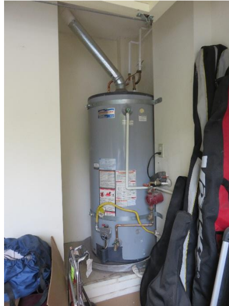
FIGURE 114. Water heater located in the garage.
