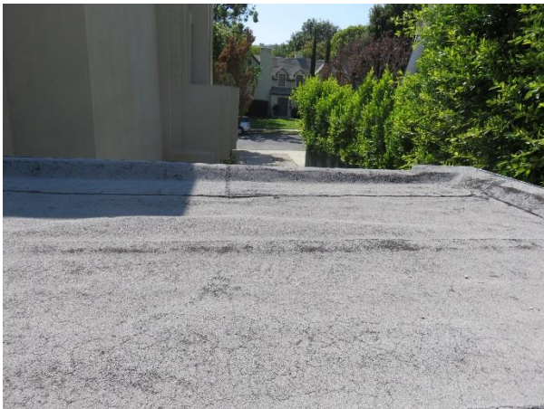
FIGURE 68. Area where the roof membrane is blistered and not bonded to the substrate.
