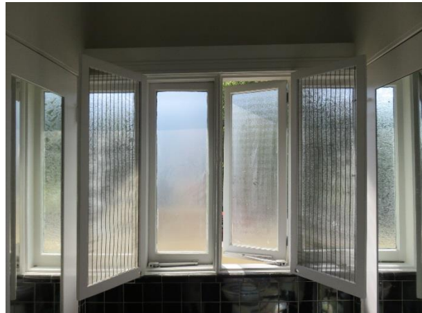
FIGURE 37. Overall view of the second floor bathroom casement window with obscure glass.
