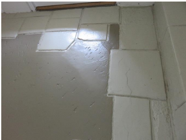
FIGURE 109. Cracks in the concrete entry slab.
