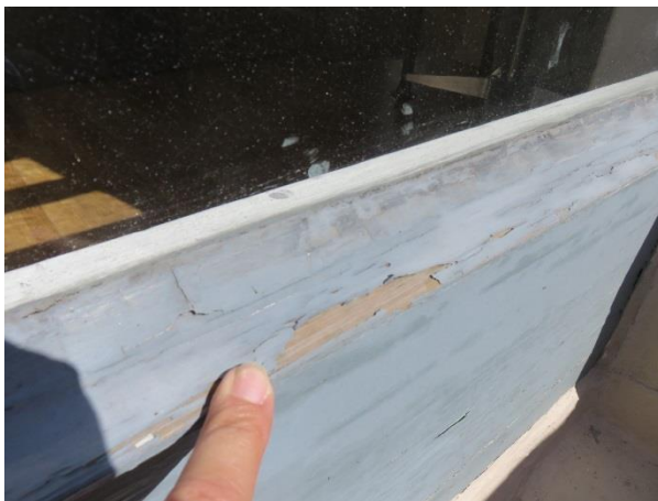
FIGURE 64. Peeling paint on the west balcony doors.
