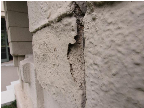
FIGURE 59. Example delaminated coating.
