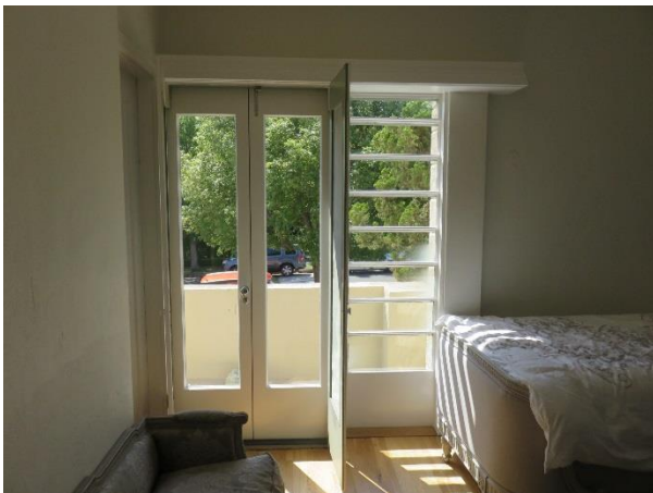
FIGURE 51. Second floor exterior door leading to the balcony on the west elevation.
