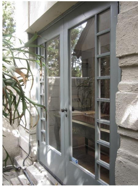
FIGURE 43. Double door on the south wall of the living room, with multi-light panels on each door.
