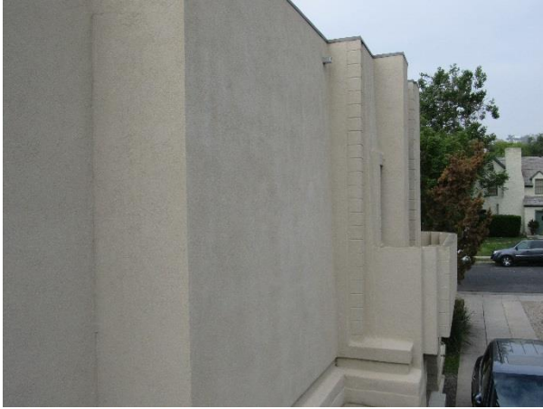
FIGURE 26. Stucco clad exterior wall at north elevation. Note the slight inward slope of the wall.
