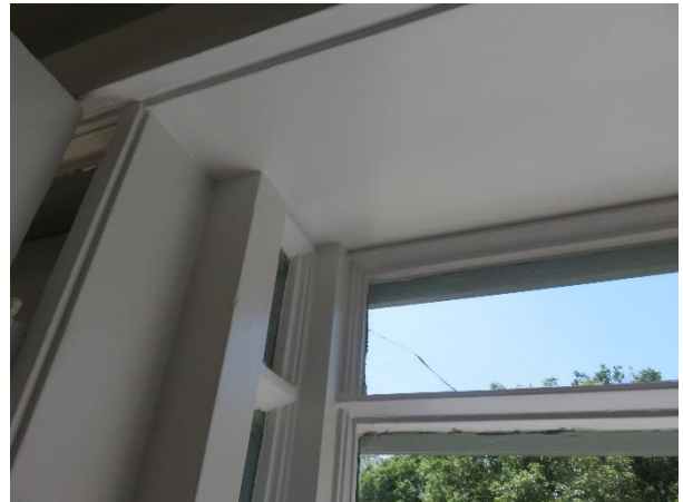
FIGURE 66. Cracked glass on the west balcony doors.
