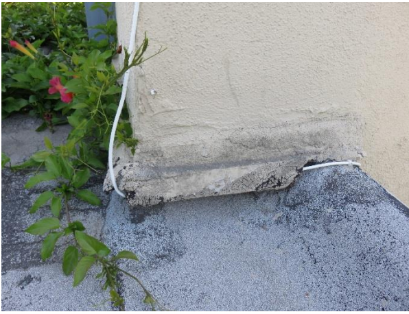
FIGURE 121. Deteriorated flashing at the roof to stucco-clad wall transition.
