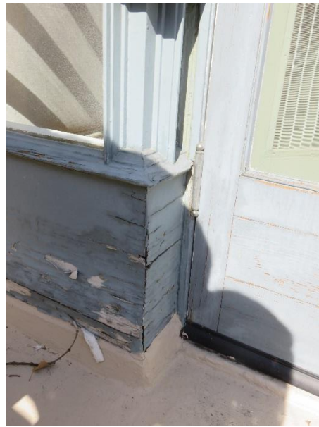
FIGURE 65. Peeling paint and deteriorated wood at the west balcony doors.
