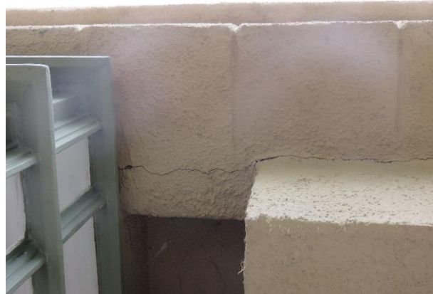
FIGURE 62. Cracking at a change of plane.
