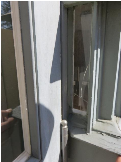
FIGURE 118. Cracked glass on the west balcony doors.
