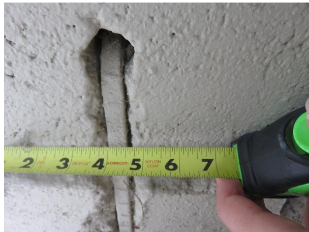
FIGURE 61. Exposed reinforcement in concrete block.
