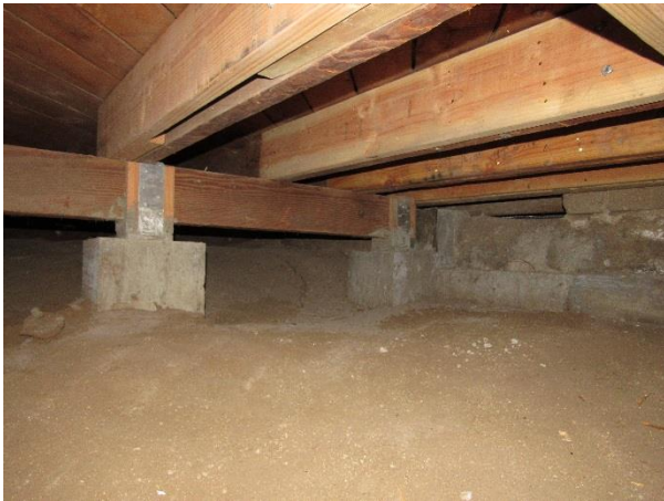
FIGURE 106. Typical wood framing at the southeast crawlspace. Note supplemental beam and strengthening of existing joists.
