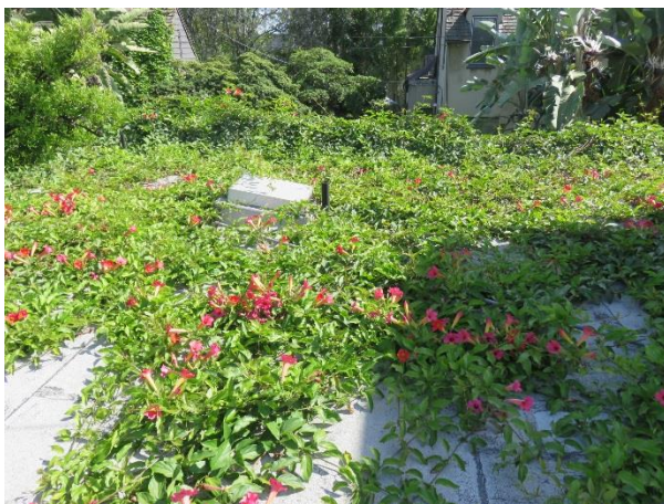
FIGURE 56. South end of the first floor roof with vines covering a large portion of the area.
