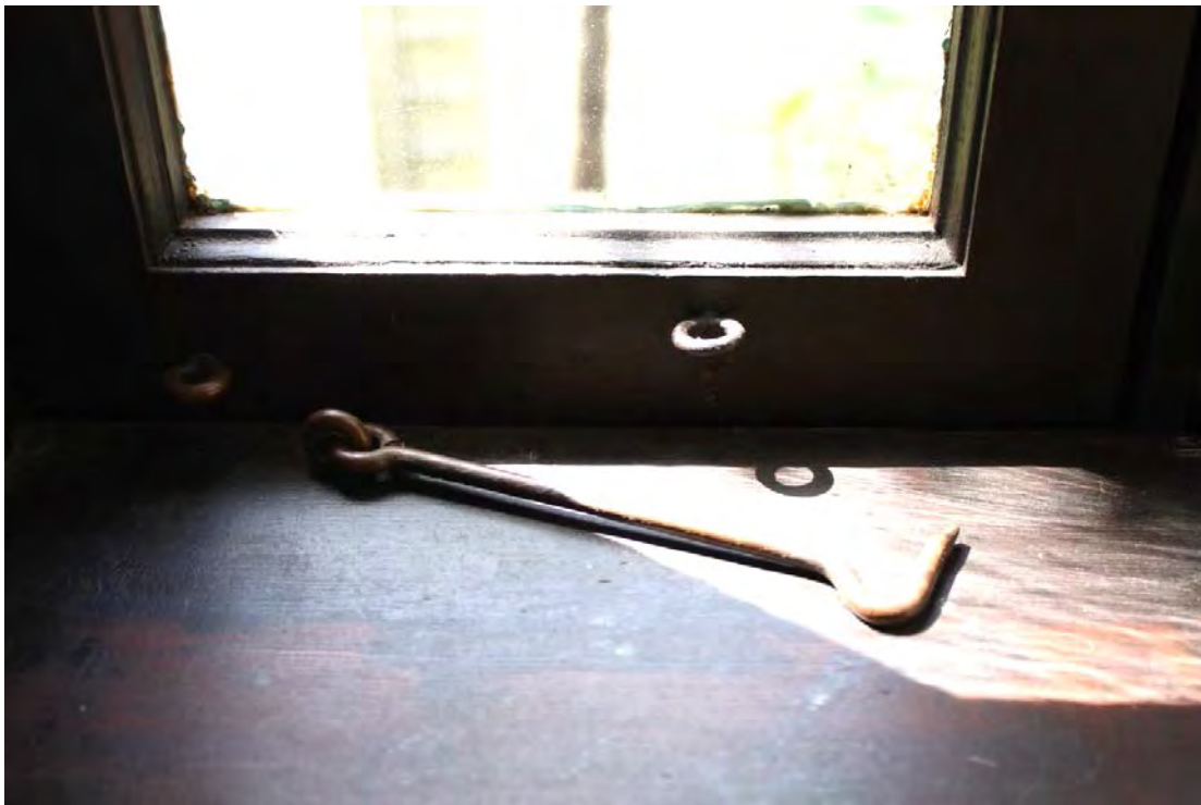
Original detail: Original studio level space of unknown use; large hook and eye casement window secure closure.
