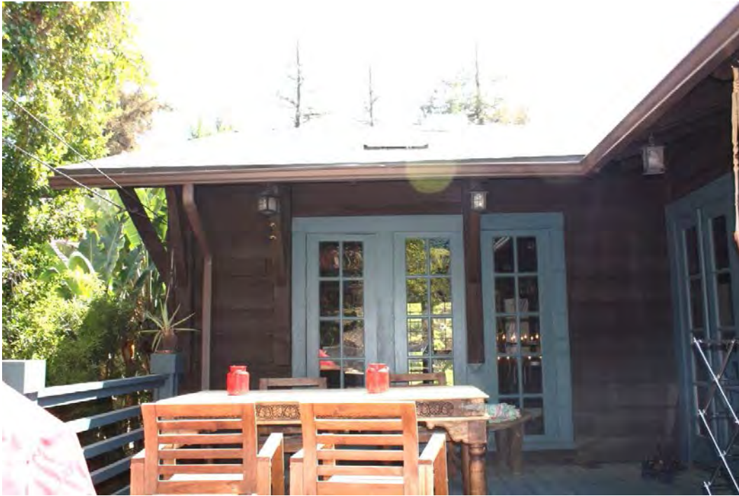
Terrace: North balustrade; east window wall with deep brackets; south wall French door ribbon; view east.
