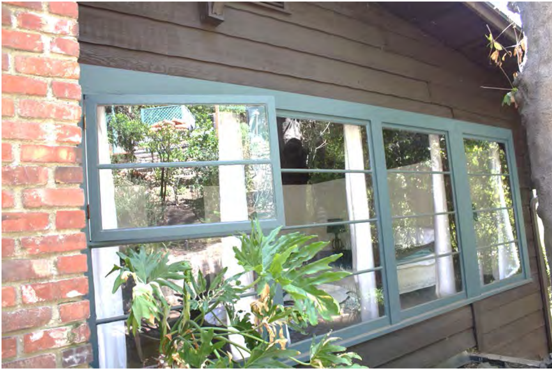
Exterior: West side of deck fireplace; master bedroom, with ribbon of casement & slider wood frame windows, west elevation with horizontal clapboard cladding, view southwest.
