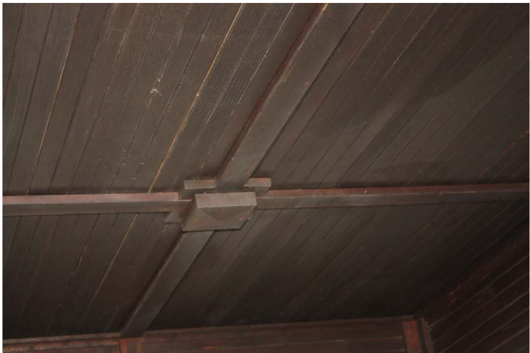
Detail: Ceiling, southeast office, second floor, tongue & groove with batten overlay accented by squares with low pyramidal accent pieces.
