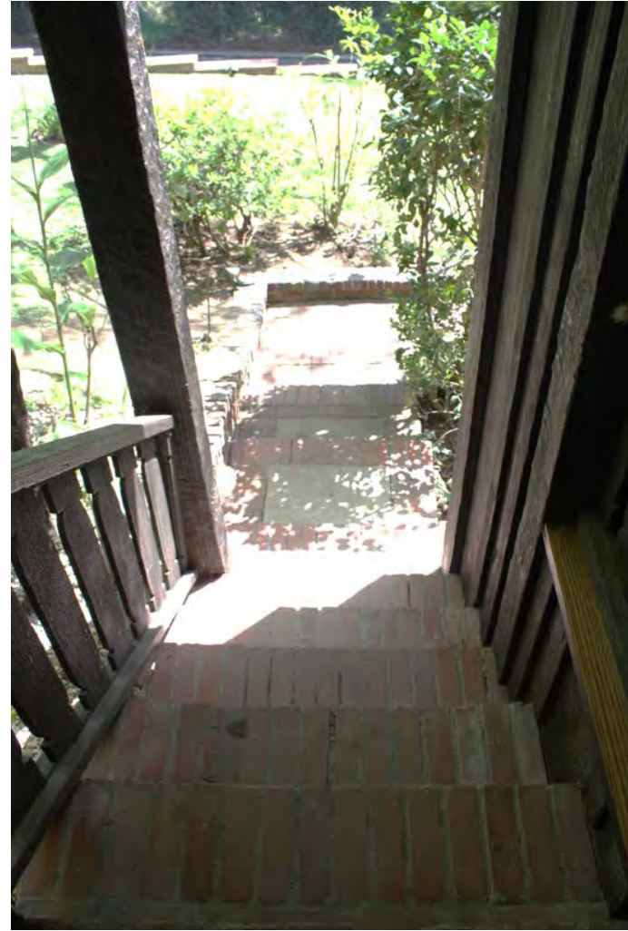
Original entry stairs leading down to lawn: North balustrade, brick steps; bat & board siding, view east.
