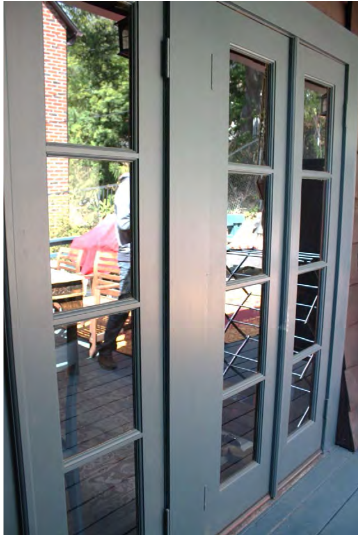
Original French doors at north elevation: Deck mirrored in glazing, view southwest.
