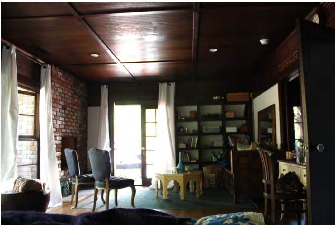
Master bedroom: West wall windows and brick fireplace; north paired French doors; wood ceiling/battens/frieze; east entry to balcony, view north.
