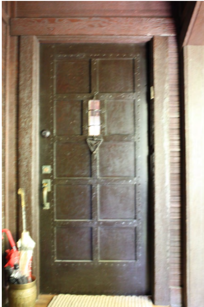
Original entry door, east façade (stock door with added panels & studded w/ hand-forged nails) and hand forged door knocker: Entry approached by open staircase & raised porch; surrounded by tongue-and-groove horizontal exterior finish; unseen porch rail at north, view west.
