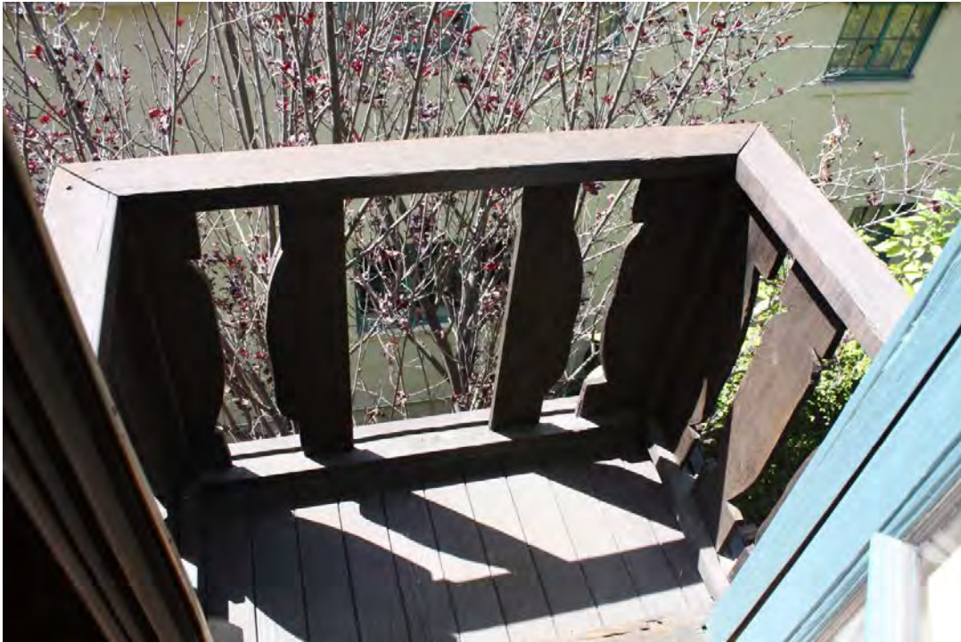
Balcony, one of two to either side of brick fireplace: Off south wall, southeast original bedroom; wood floor; wood shaped banisters in balustrade, view south.
