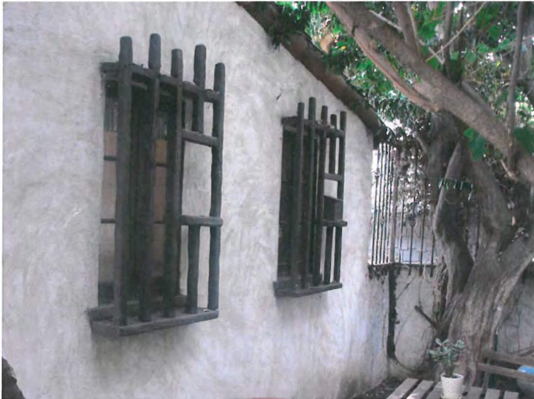
Casa de Mi Sueño, front window grilles, 3820 San Rafael Avenue, February 26, 2014 (photograph by Charles J. Fisher)
