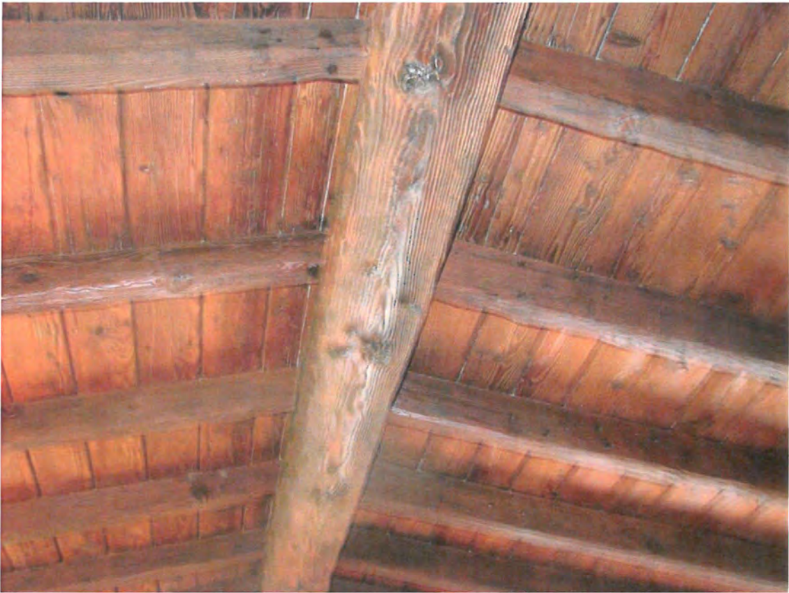
Casa de Mi Sueño, Living room ceiling, 3820 San Rafael Avenue, February 26, 2014 (photograph by Charles J. Fisher)
