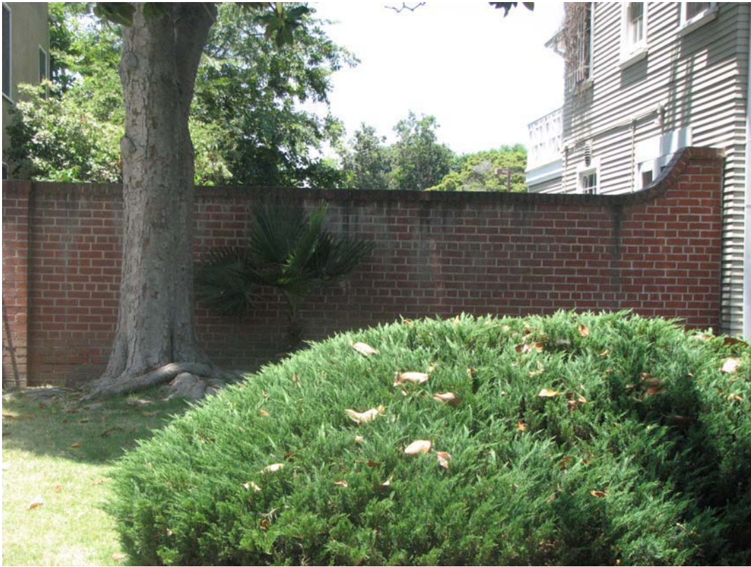
Heerman Estate, one of several brick walls on property, 525 S Van Ness Avenue (Photograph by Charles J. Fisher)
