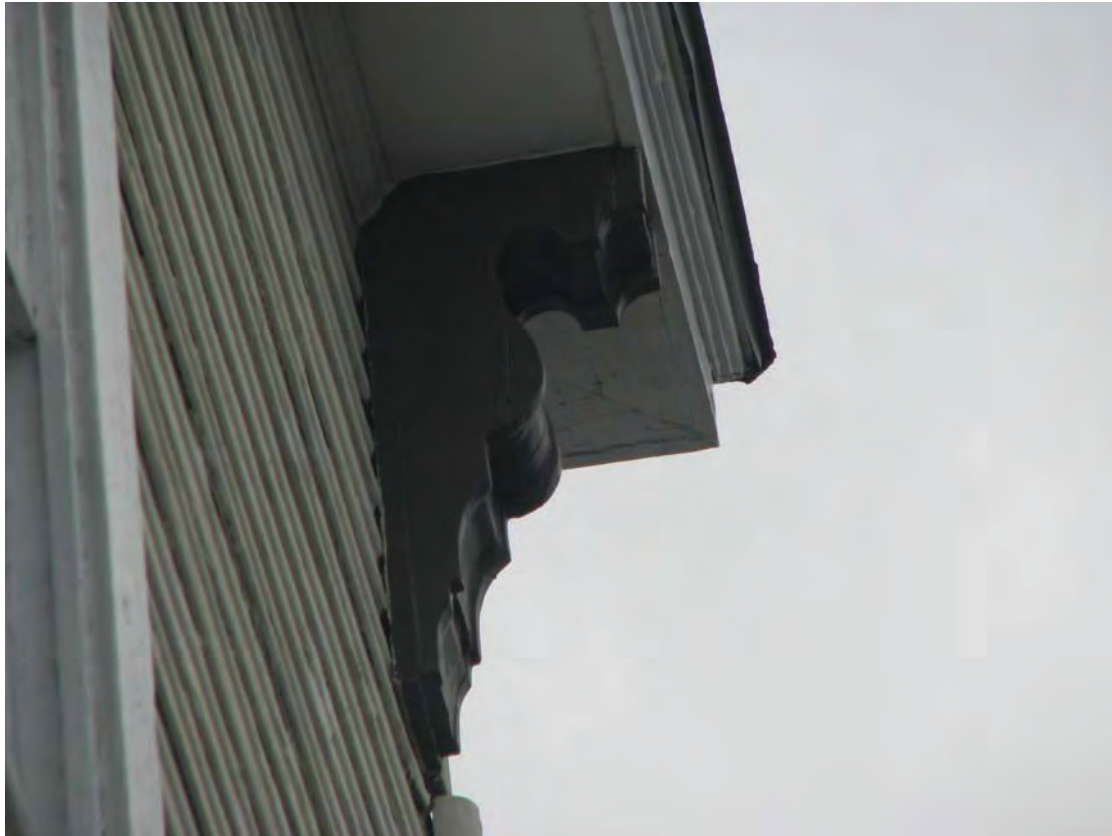
Restovich House, roof corbel, 1001 Everett Street, September 19, 2014 (Photograph by Charles J Fisher)
