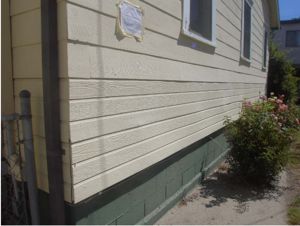
15. Siding detail, with 1937 asbestos siding above and two sections of fabricated, three-course siding below. South elevation. View Northeast
