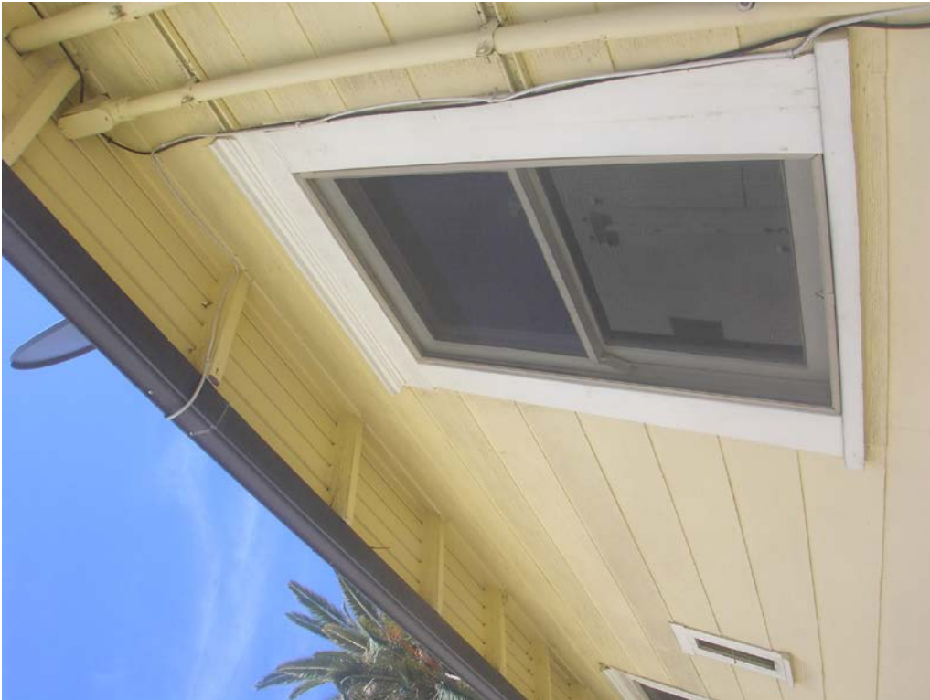
14. Rear elevation detail, with double-hung window and exposed rafters and roof boards at eaves. View: Northeast
