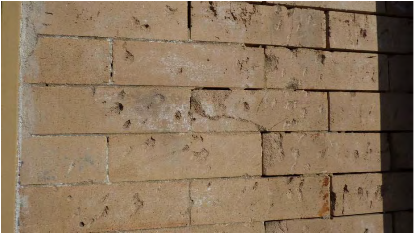
Figure 19. Damaged pressed brick on front façade, possibly from sandblasting in 1994, view north (PCR 2015)
