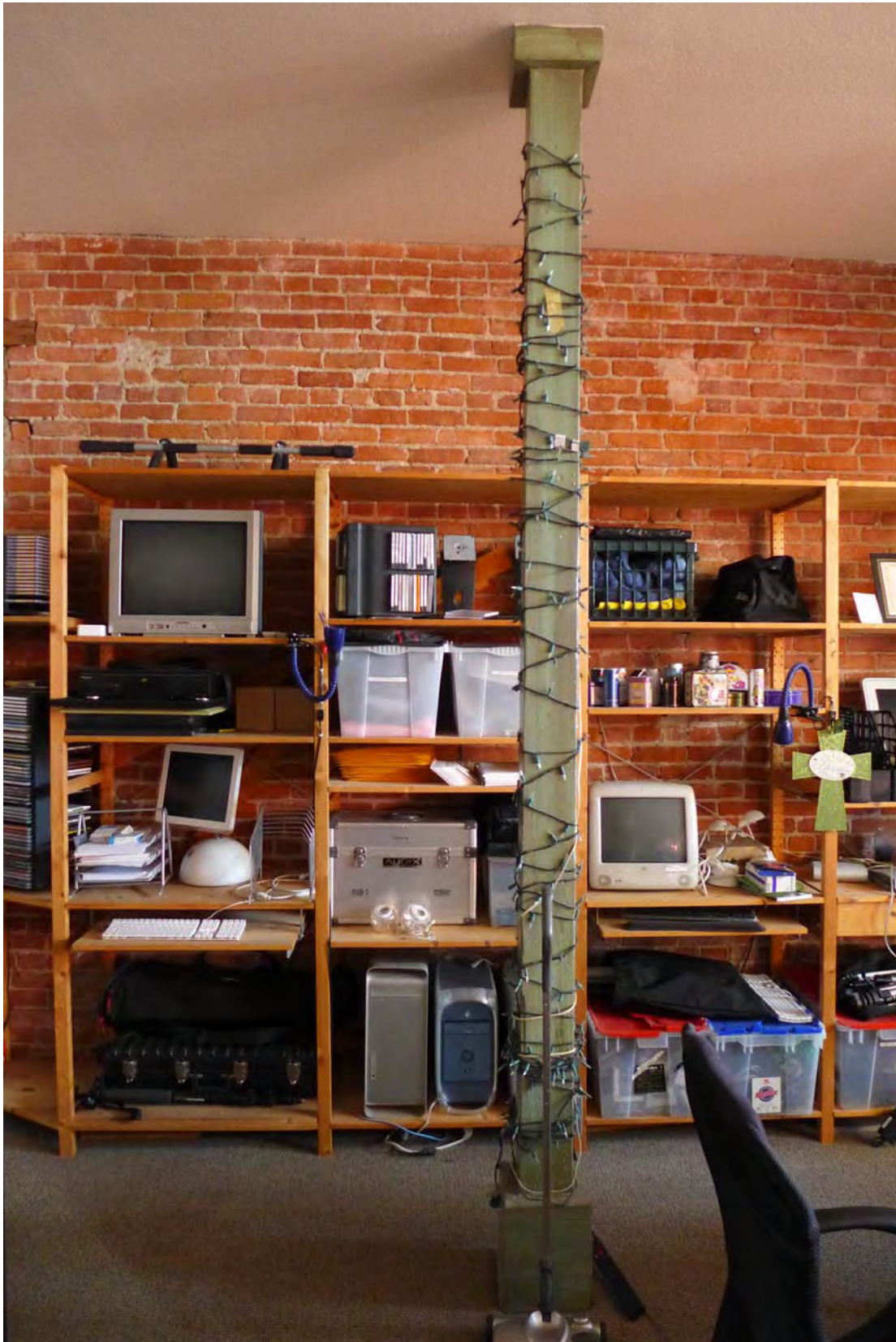
Figure 36. Wood support beam on the eastern side of the first floor interior, possibly original (PCR 2015)
