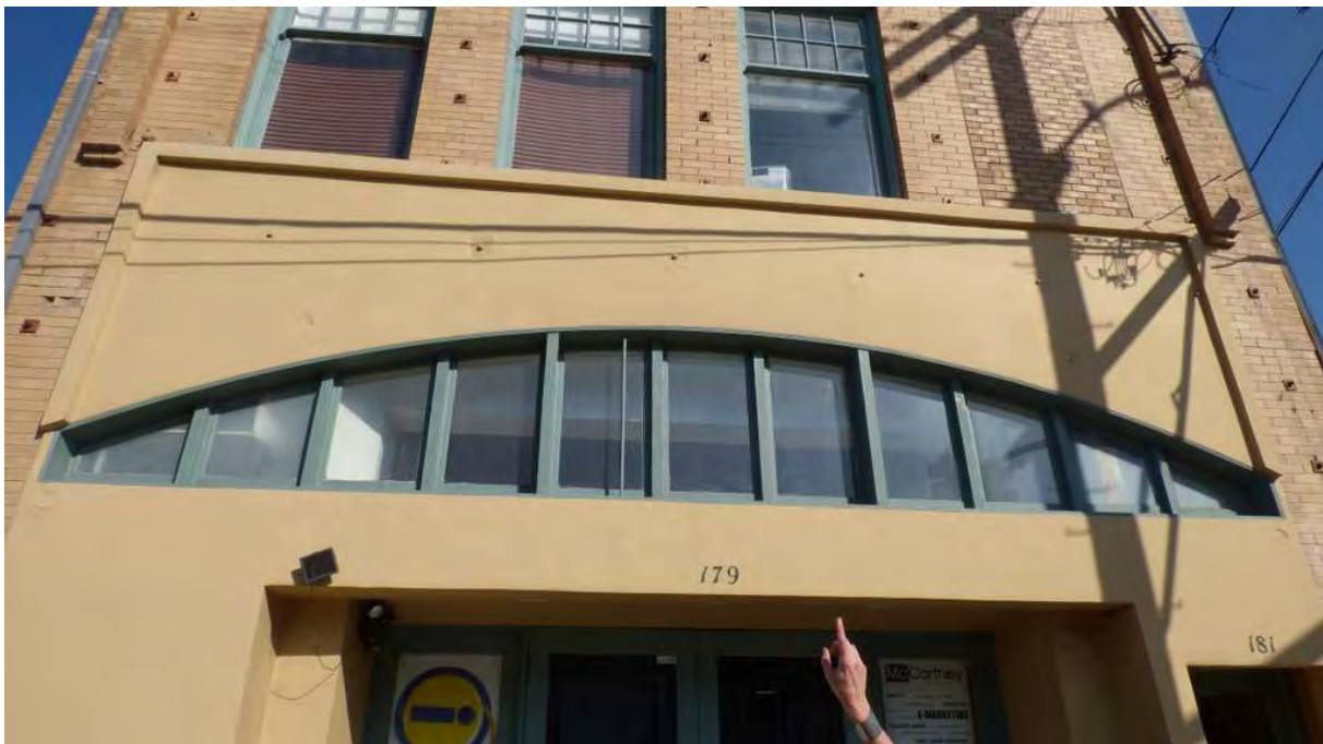
Figure 24. Concrete (alteration) covering 1933 wood frame storefront, with signage removed and alterations to framing of arched transom windows. Additionally, the windows are partially blocked by interior alterations on either end (alteration). View north (PCR 2015)
