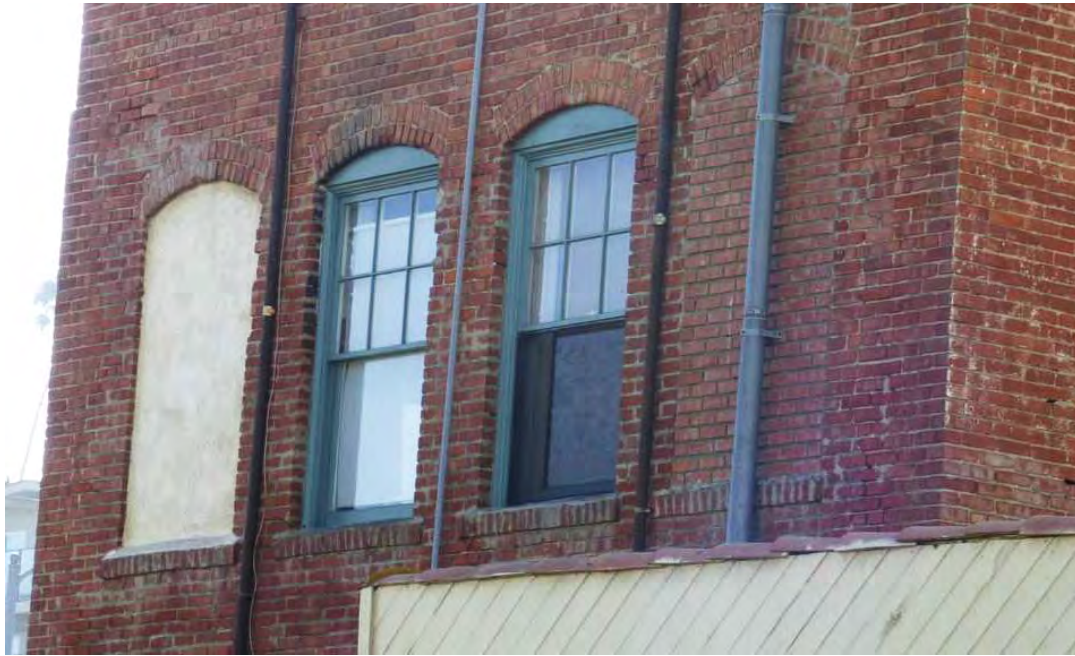
Figure 29. Detail of rear (north) elevation showing two, six-over-one casement windows surmounted by brick arches flanked by two filled in window (alteration, far left and far right) (PCR 2015)
