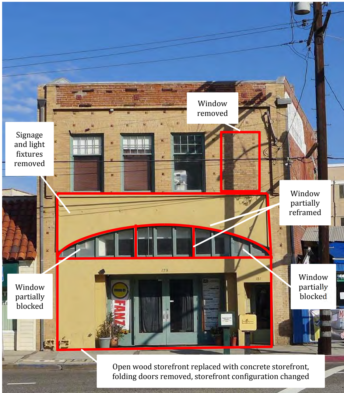
Figure 48. Alterations to historic appearance of the subject property from the secondary period of significance 1933 to 1966 (PCR 2015)
