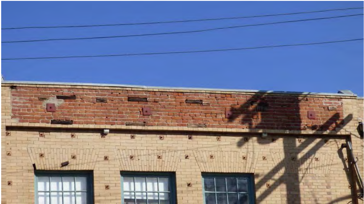
Figure 21. Exposed red brick where cornice and parapet were removed in 1933, view north (PCR 2015)
