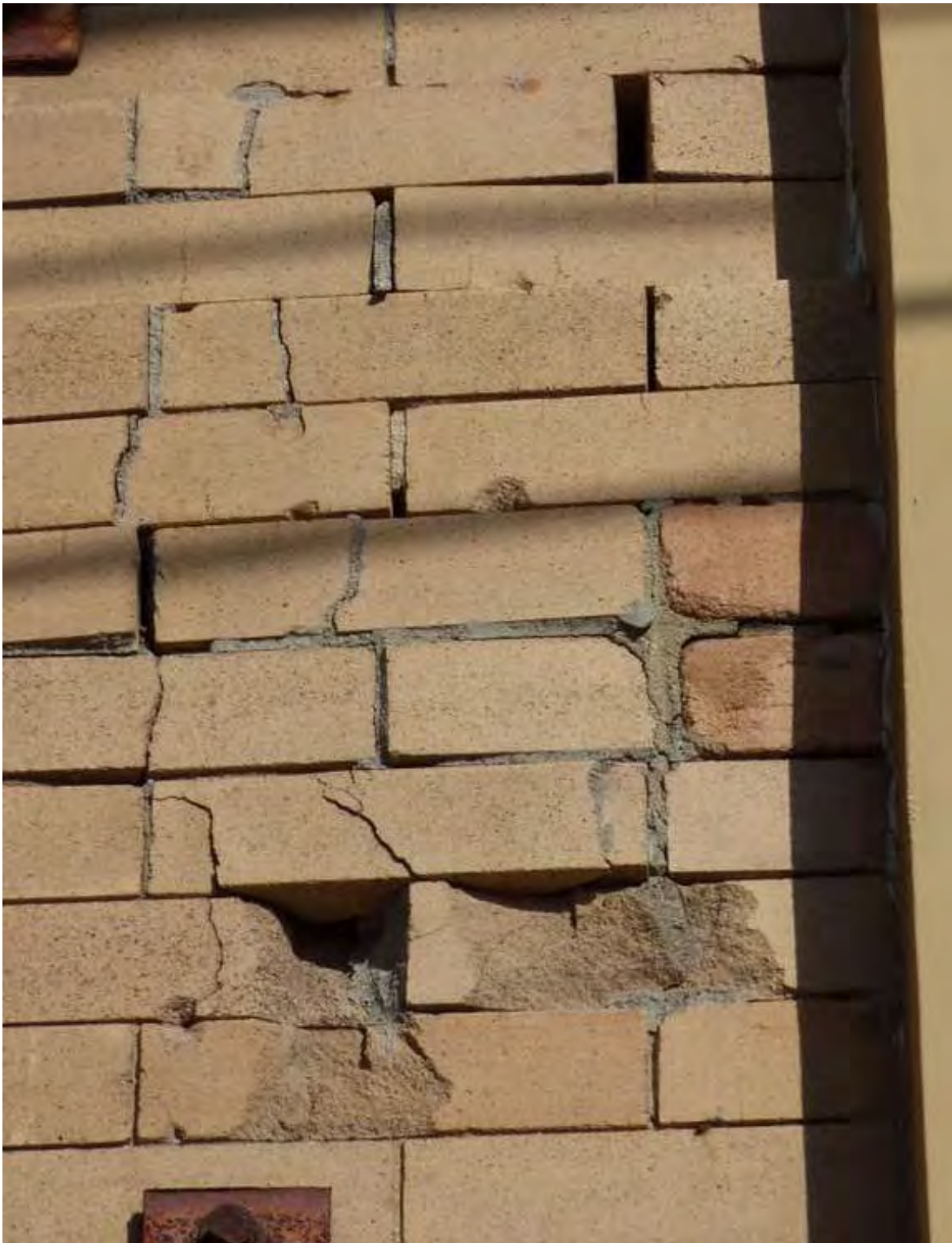
Figure 20. Cracked and damaged brick on front façade, with chunks of brick missing, view north (PCR 2015)
