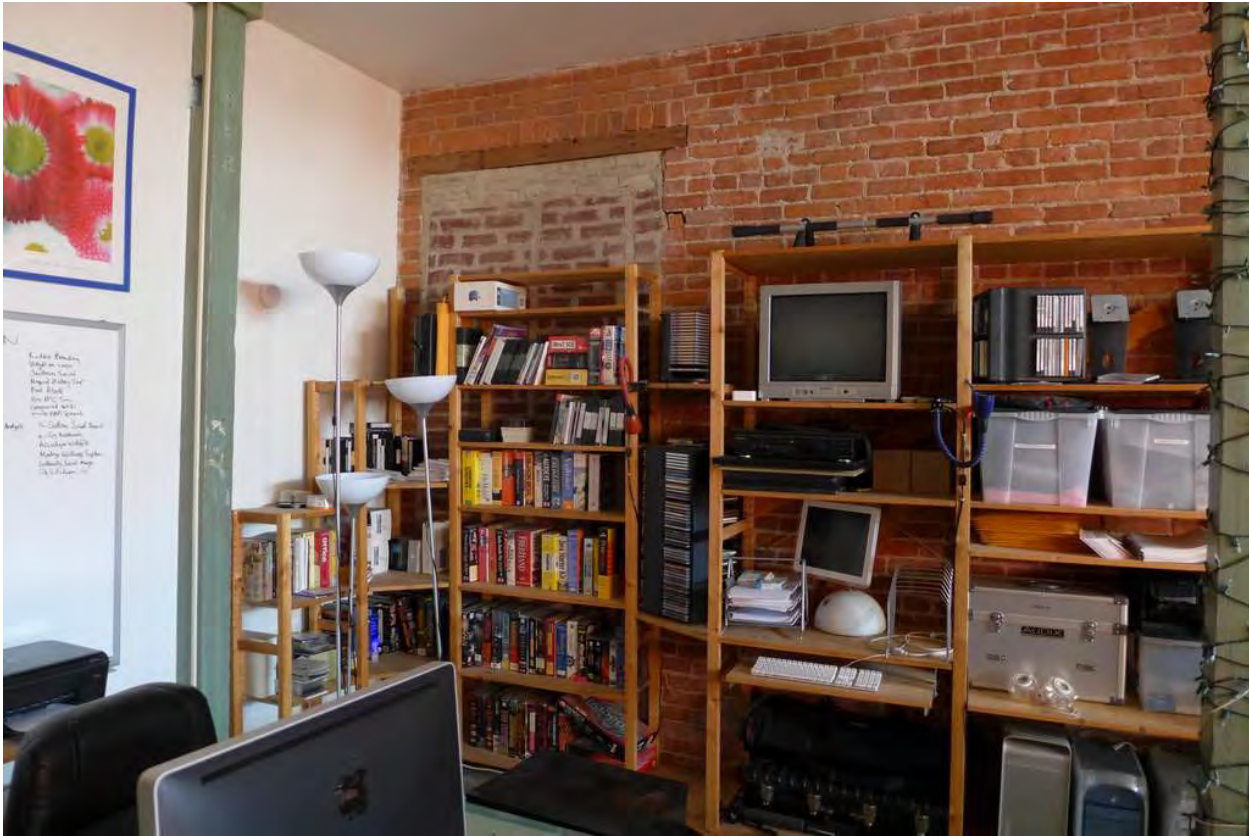
Figure 35. Bricked in window opening (alteration) with wood lentil on the east wall of the first floor (PCR 2015)
