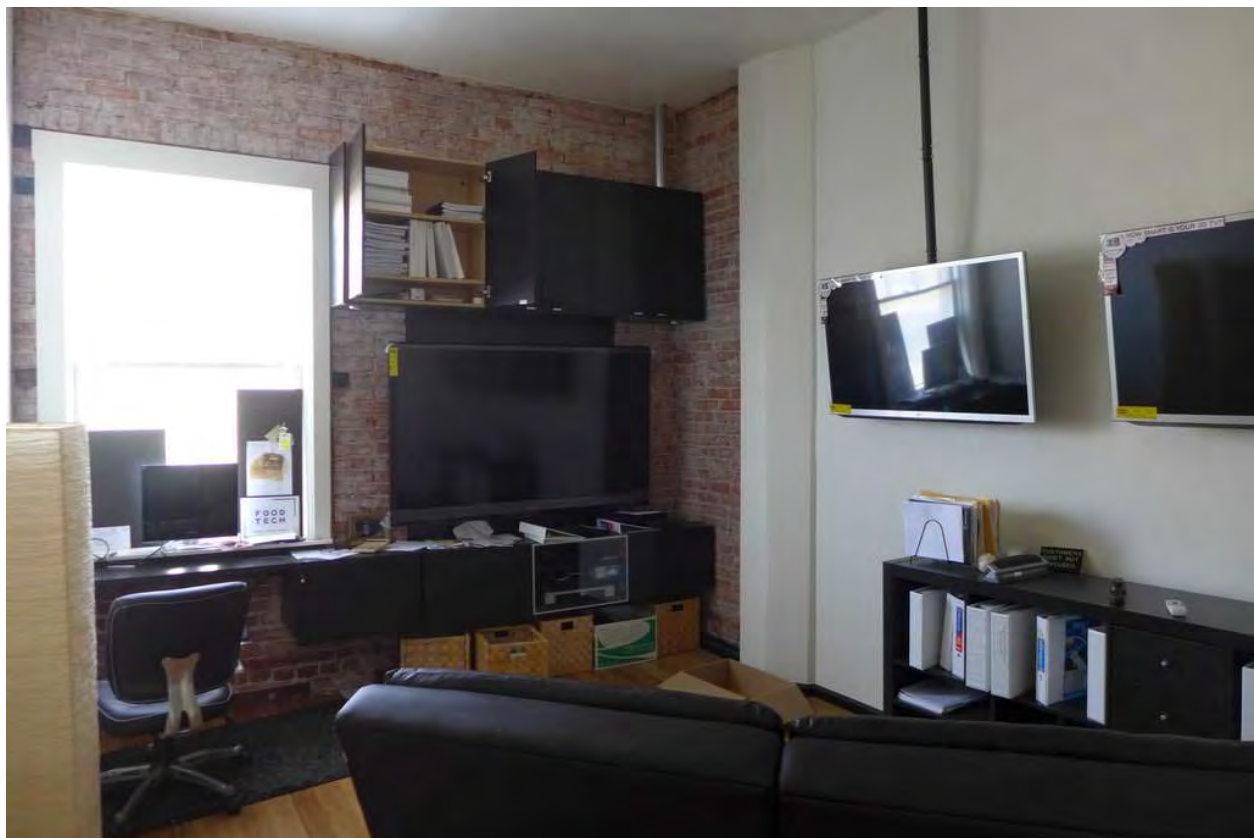
Figure 46. Exposed brick in a second floor office unit, brick has a white discoloration (PCR 2015)
