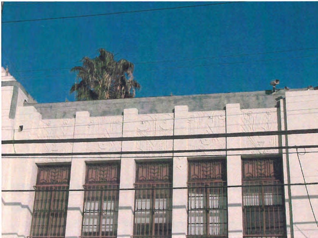
Redwine Building, parapet, 1618 N. Las Palmas Avenue, February 5, 2015 (photograph by Charles J. Fisher)
