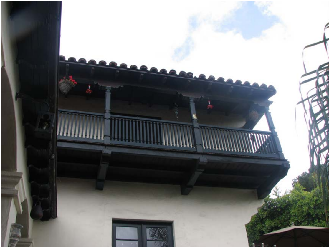
Durex Model Home, second floor balcony, 3410 Amesbury Road, April 11, 2012 (Photograph by Charles J. Fisher)
