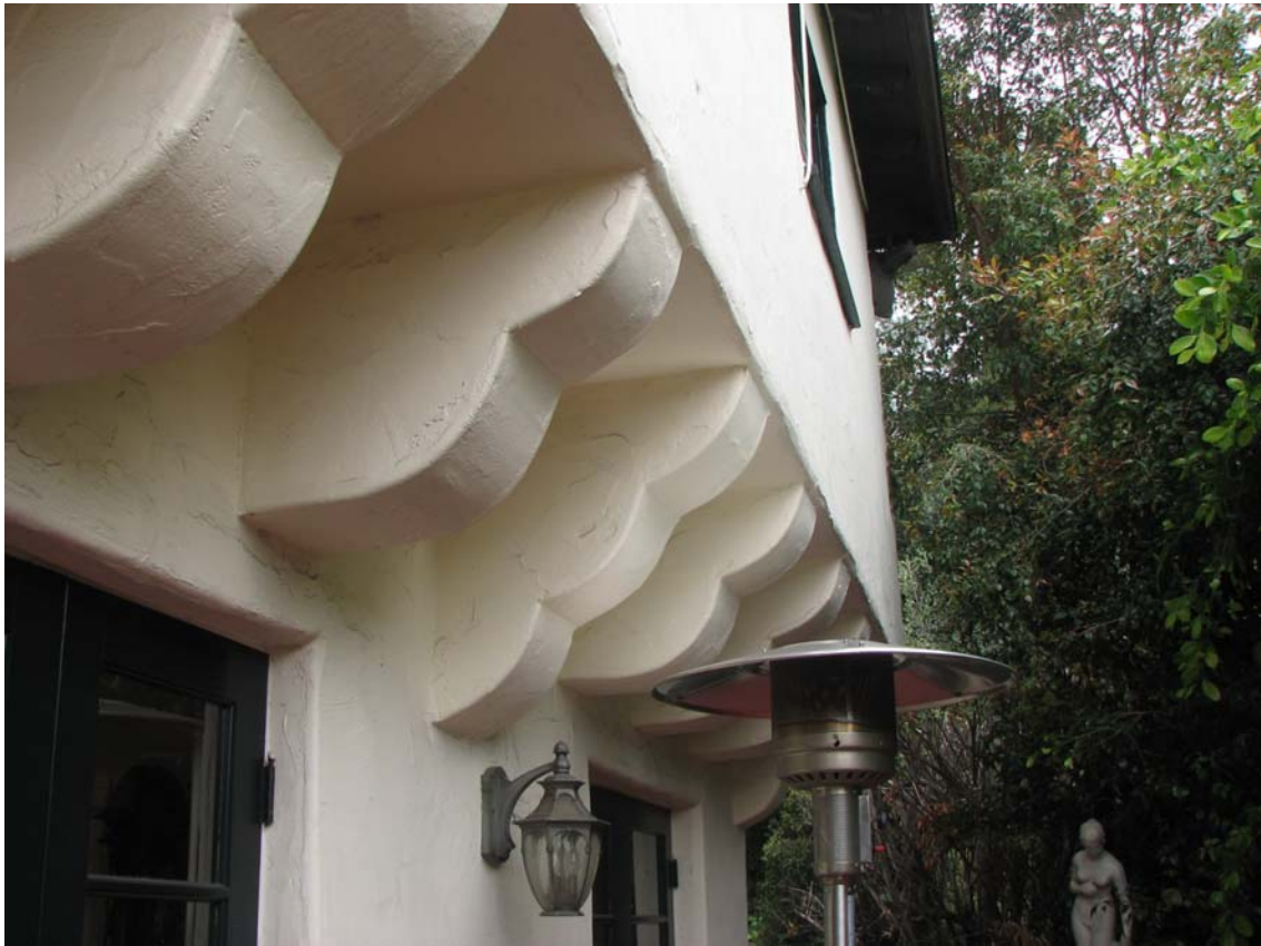
Durex Model Home, corbels, 3410 Amesbury Road, April 11, 2012 (Photograph by Charles J. Fisher)
