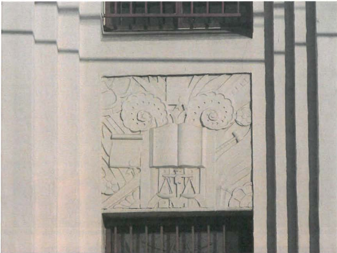
Redwine Building, panel above entrance, 1618 N. Las Palmas Avenue, Feb. 5, 2015 (photograph by Charles J. Fisher)
