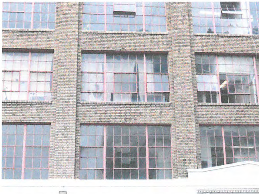
Steel sash on upper façade are original, and in fair condition. Note awning operation of center sash
