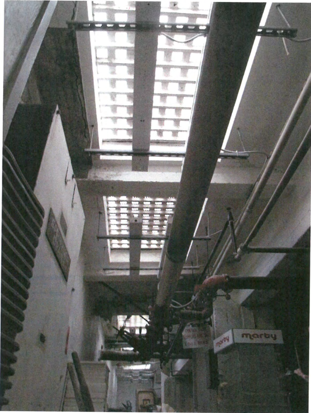
Figure 22. View looking up at the vault lights along the western wall of the basement level.
