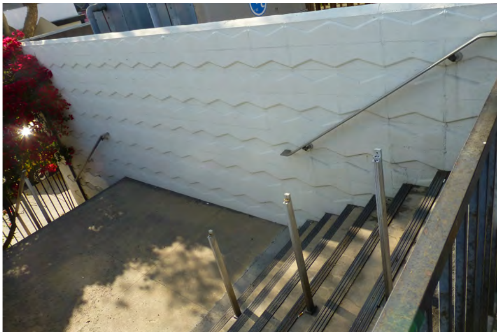
Exterior Set of Stairs to Secondary Entrance, southwest corner, view northwest (2016) Steve Luftman
