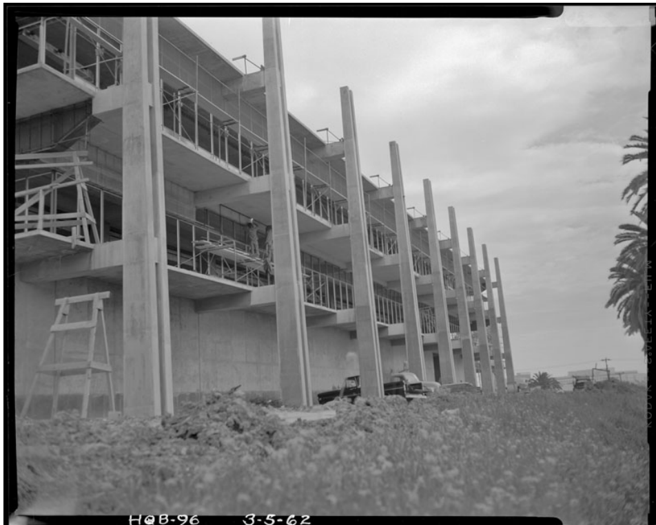
6. Metropolitan Water District Headquarters Campus under construction, Original Building Sunset wing, c. 1962
