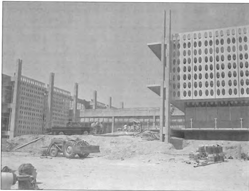
Figure 4: East entry during construction, note shaping of grassy knoll, view west (MWD archives, 1962)
