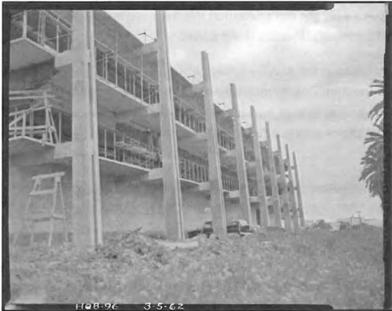
West Elevation 1962 – This is basically how the building looks now once the owner removed the Sun screens and guard rails.
