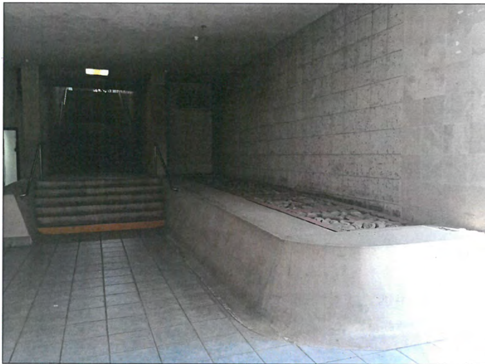
Figure 26: Building 2, interior, first floor, view north, note concrete planter at right (Snow, 2016)
