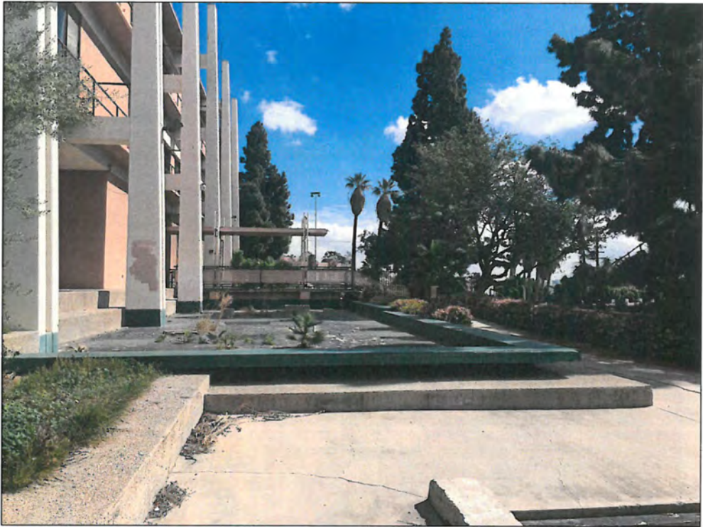
Figure 9: Building 1, south elevation, view east, note empty and altered water features (Snow, 2016)
