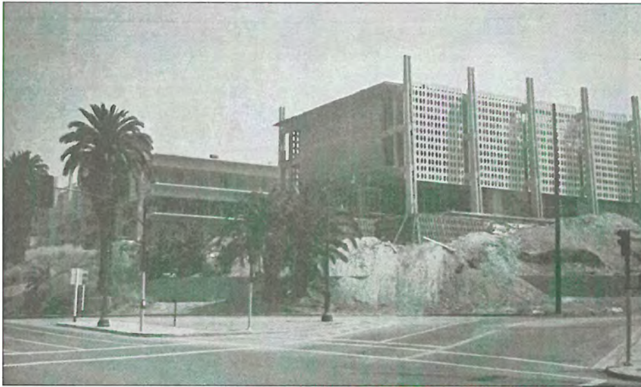
Historic Photograph 16: Building 3a (left) and Building 1 (right) under construction, view southeast from Sunset Boulevard (1962, MWD Annual Report, caption reads, “Pictured...is a recent view of the Metropolitan Water District’s new headquarters building at 1111 Sunset Boulevard. Construction is now nearly 90 percent complete.”)
