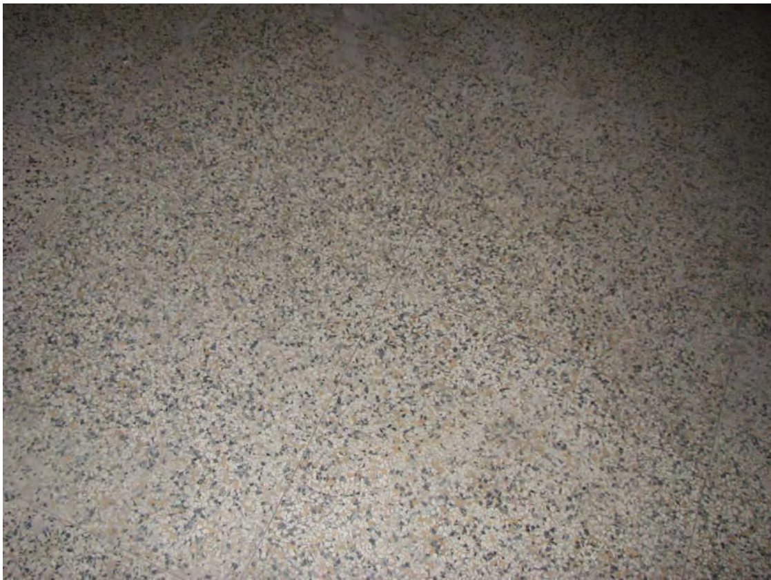
F & W Grand Silver Building, terrazzo flooring, 537-41 S. Broadway, July 23, 2015 (Photograph by Charles J. Fisher)
