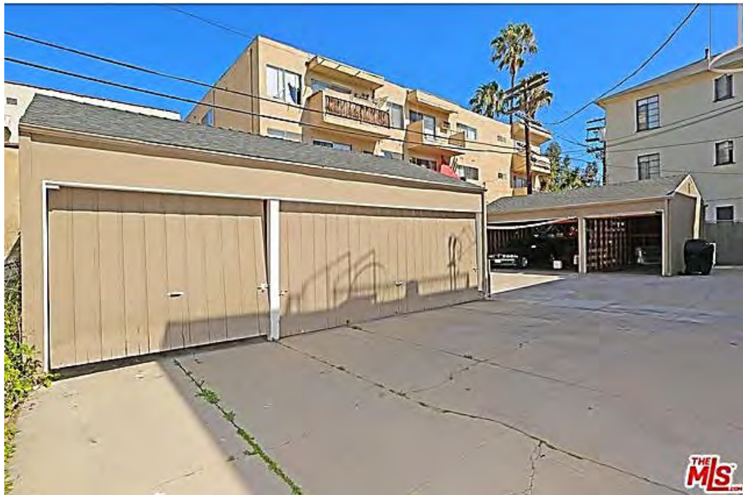
Garages at east of apartments, view southeast. Note: Condition of pavement. Photograph courtesy of the MLS, July 2015.
