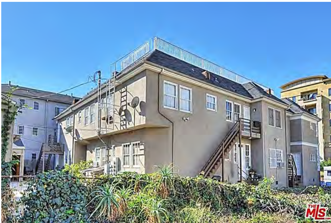
View to east and north elevations, view southwest, with egregious white railing at roof. Photograph courtesy of the MLS 2016.
