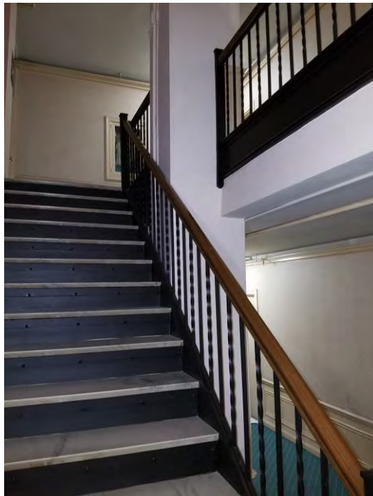
Stairway 2 accesses the upper stories. The marble stair treads and balustrade with wood bannister are original and should be retained. The railing does not meet current code requirements. A variance may be required to avoid future modifications of the railing, or the potential to enclose the stairwell, which would have a major impact on the character of the corridors, and the interior in general.
