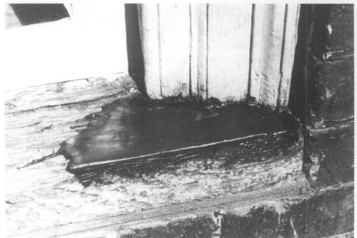
Figure 5. This illustrates a two-part epoxy patching compound used to fill the surface of a weathered sill and rebuild the missing edge. When the epoxy cures, it can be sanded smooth and painted to achieve a durable and waterproof repair. Photo: John H. Myers
