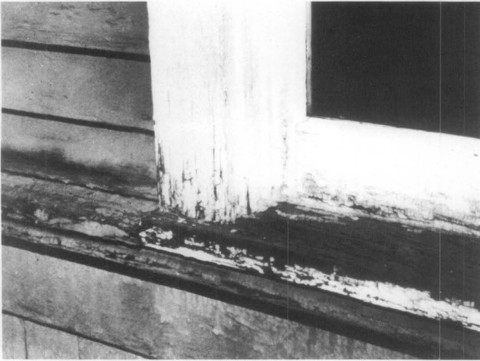
Figure 3. Deterioration of poorly maintained windows usually begins on horizontal surfaces and at joints where water can collect and saturate the wood. The problem areas are clearly indicated by paint failure due to moisture. Photo: Baird M. Smith, AIA
