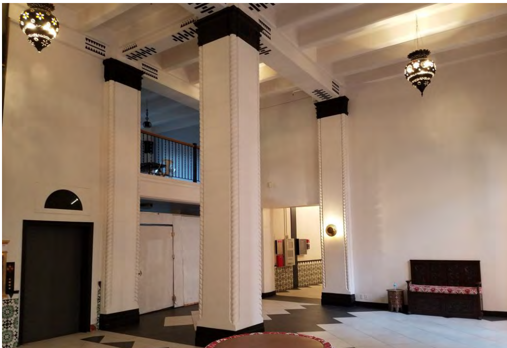
Lobby, as modified, Fall 2016. Future changes include installation of a new desk area in rear corner (now plywood) with millwork based on historic photo, (prior page, same view) and cabinetry in original cafe/retail space (still extant).
