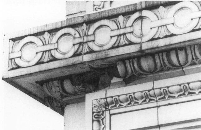
Figure 7. Material Spalling. Excessive expansion of the porous tile body caused by water and freezing temperatures produces major material spalling, a situation often difficult to repair.
