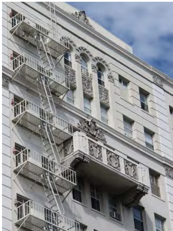
Upper façade ornamentation and balconies, typical on the primary elevations. All of these components need periodic inspection for cracks and any weakening of the attachments.
