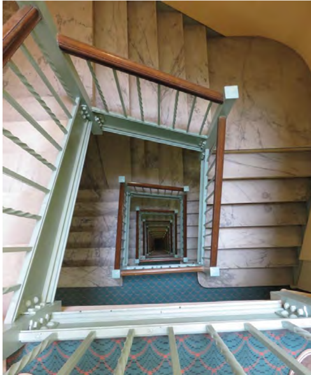
Stairway 1 winds through the upper stories. The marble stair treads and balustrade with stained natural wood bannister are original and should be retained.
