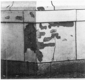
Figure 6. Glaze Spalling. Blistering of the glaze, like crazing, is the result of the increase in water in the porous clay body and the subsequent destruction of the glaze as a result of water migration and pressure. Glaze spalling may also be caused by deterioration of metal anchors behind the terra-cotta unit.
