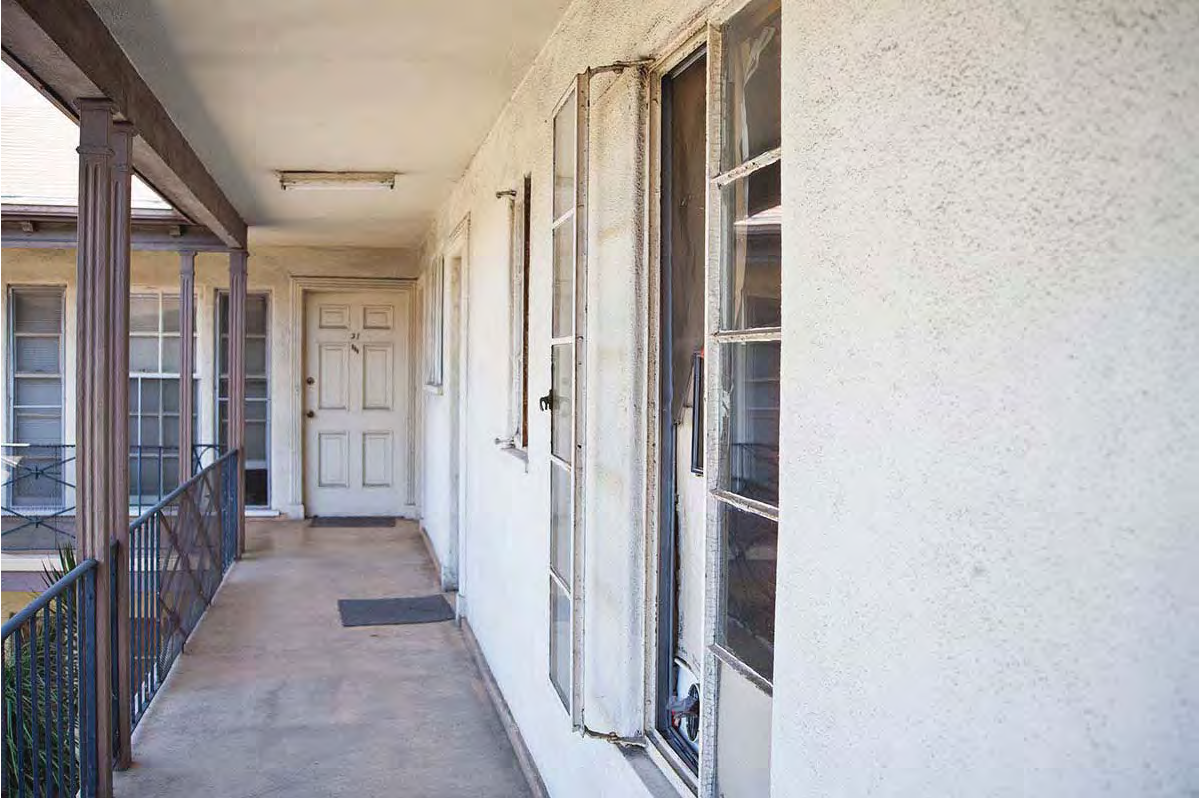
Selma Las Palmas Courtyard Apartments, 1535 N Las Palmas Avenue, September 11, 2017 (Photograph by Susan Hunter)
