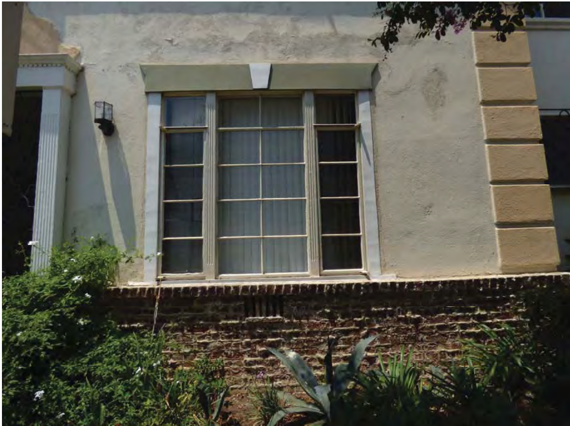
Selma Las Palmas Courtyard Apartments, window & bulkhead, 1545 N Las Palmas Ave, July 13, 2017 (Photo by Charles J. Fisher)
