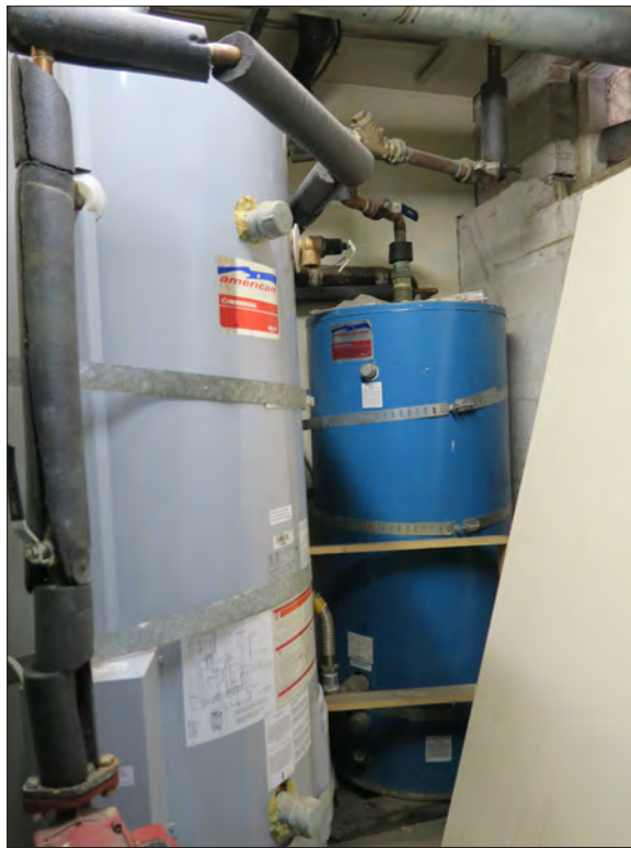
Image 38: Basement, mechanical equipment (Chattel, 2017)
