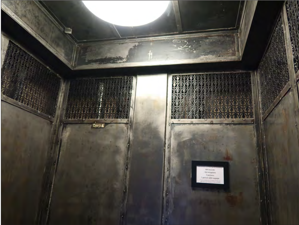
Image 19: Elevator cab interior (Chattel, 2017)
