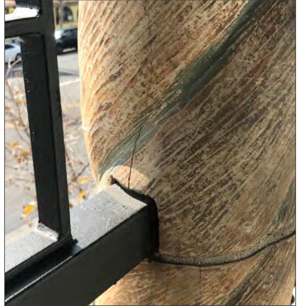
Detail of railing connection at terra cotta column. Note vertical crack at column (ARG, 2018)
