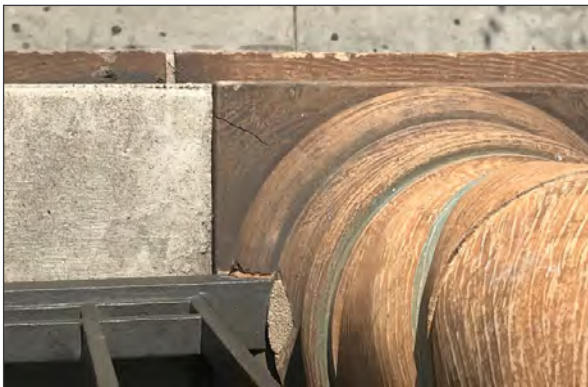
Crack at base of terra cotta column (ARG, 2018)
