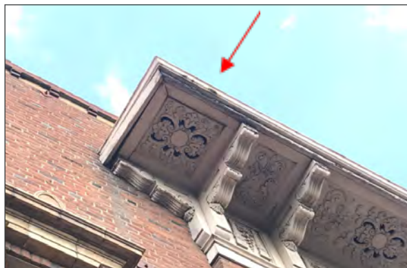
Deteriorated and loose trim at end of cornice, southeast elevation. Also note vents at cornice soffit (ARG, 2018)
