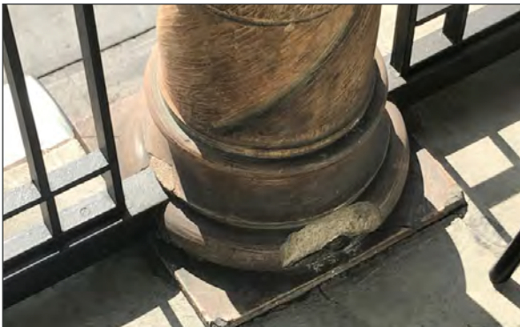
Large spall at balcony side of terra cotta column, and previous patch at railing connection (ARG, 2018)
