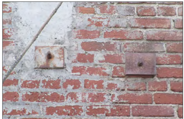
Detail of seismic plates and anchors at second floor level, northwest elevation. Note surface corrosion (ARG, 2018)
