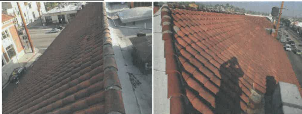
The roofing material on the sloped roof is made of clay tile.
