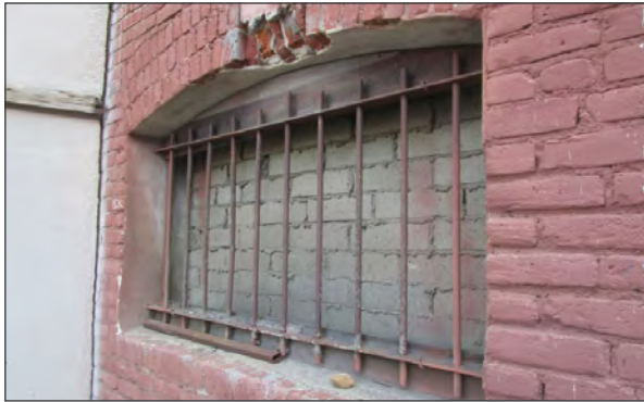
Damaged brick at window opening, southwest elevation (ARG, 2018)
