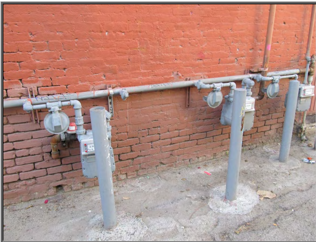
Photo 20: Gas service meters - note automatic shut-off valve at meter on the left.
