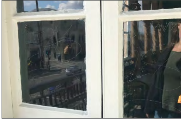
Paired wood casement window at west end of second floor balcony; note scratched glass pane (ARG, 2018)
