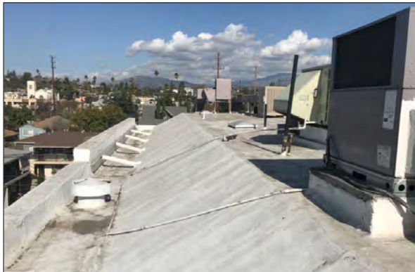
Membrane roof, view northwest. Note bracing at parapets and rooftop units (ARG, 2018)
