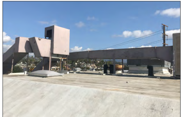
Membrane roof, view north. Note mechanical equipment and ductwork for restaurant kitchen (ARG, 2018)
