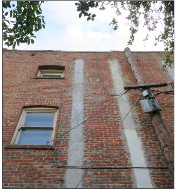
Detail of northwest elevation. Note windows with brick sills, and bands of mortar (ARG, 2018)
