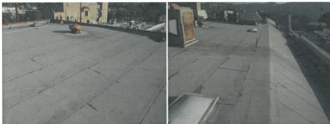
The roofing material on the low sloped roof is rolled sheet composition roofing with a granular surface.
