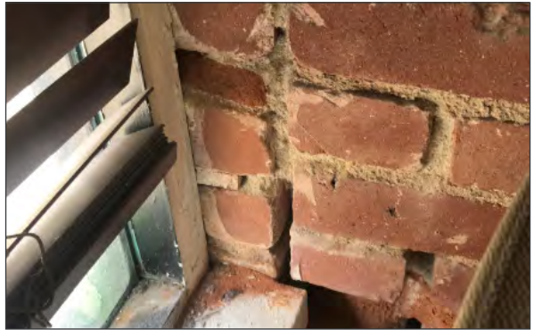
Deteriorated brick and mortar at interior side of brick wall, southeast building corner (ARG, 2018)
