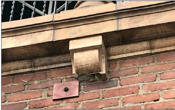
Spall damage at terra cotta unit, southeast elevation. Damage may have occurred during installation of adjacent seismic plate/tie rod (ARG, 2018)
