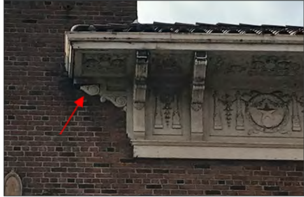
Deteriorated cornice at northeast elevation; also note loose bracket at wall (ARG, 2018)
