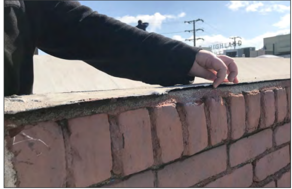
Deteriorated mortar joints at top of parapet wall (ARG, 2018)
