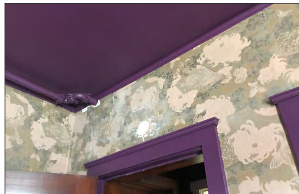
Southeast parlor, damage to wallpaper over entrance; note plaster patches (ARG, 2018)
