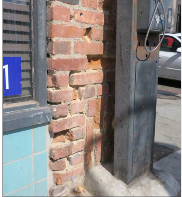
Deteriorated and missing brick at southeast corner (ARG, 2018)
