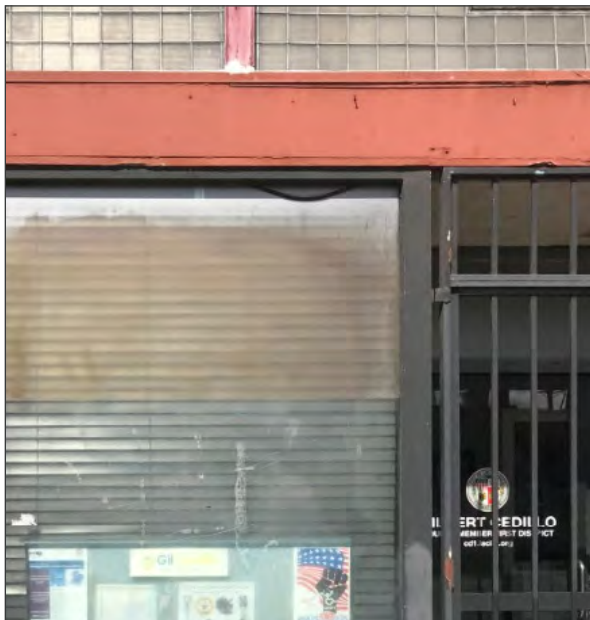
Detail of storefront, 5577 North Figueroa Street; note loose gaskets and deterioration (ARG, 2018)
