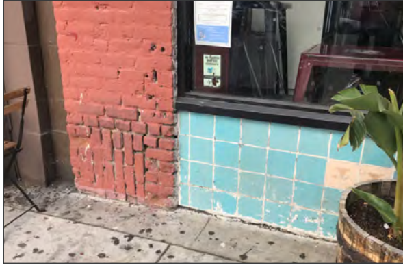
Open mortar joints at base of wall, northeast elevation (ARG, 2018)
