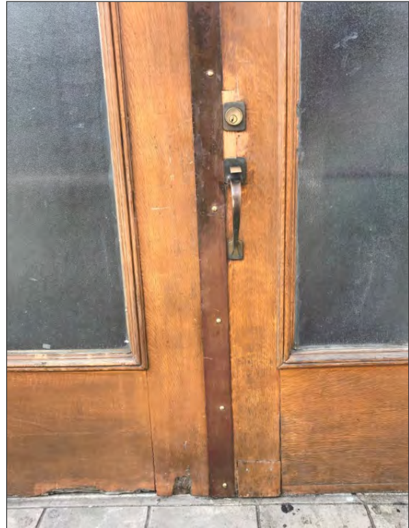
Damage and previous repairs at wood doors, northeast elevation (ARG, 2018)
