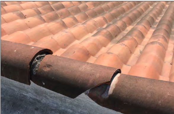
Chipped and broken ridge coping tile along northeast elevation (ARG, 2018)
