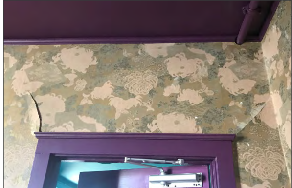
Northwest parlor, damage to wallpaper over entrance (ARG, 2018)
