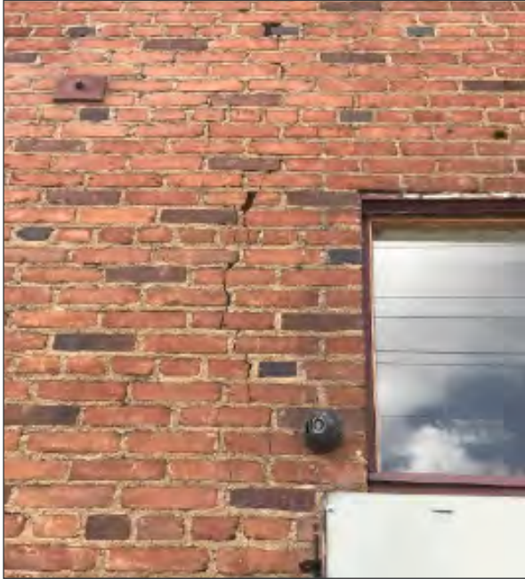
Crack at brick masonry, northeast elevation (ARG, 2018)
