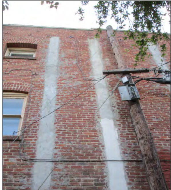
Seismic wall anchors and braced framing at exterior URM wall, northwest elevation (ARG, 2018)
