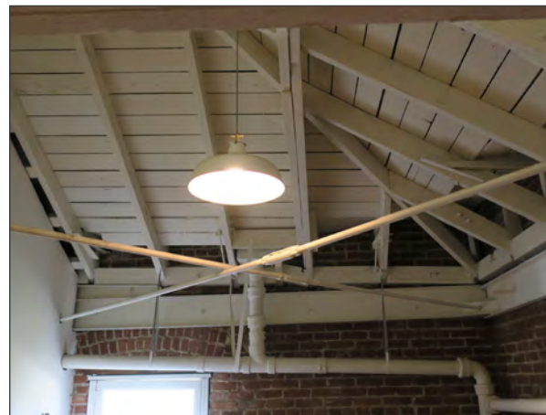
Exposed wood bowstring trusses and roof framing at northeast end of third story (ARG, 2018).
