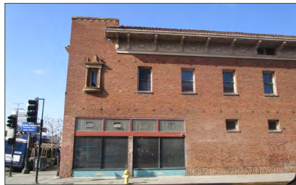
Current storefronts at east end of northeast elevation; note original transoms remaining (ARG, 2018)
