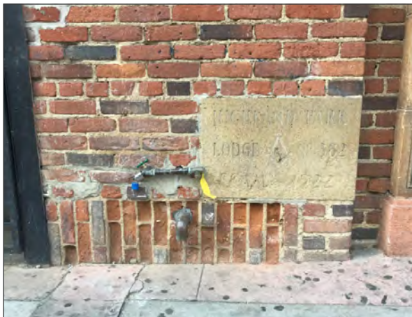
Eroded/deteriorated brick at base of building wall, northeast elevation (ARG, 2018)
