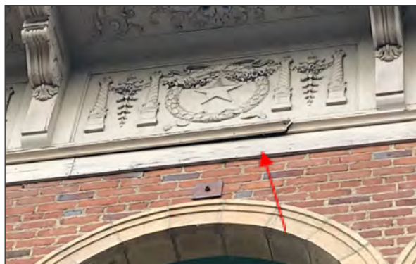
Loose trim at southeast elevation frieze panel (ARG, 2018)
