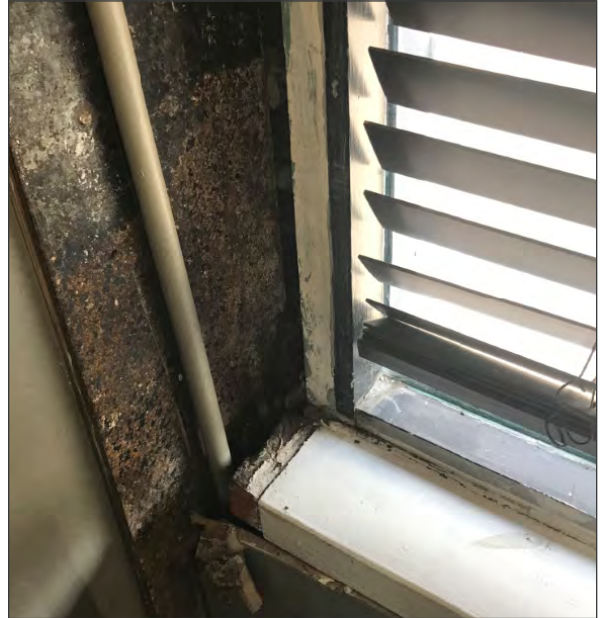
Corrosion at steel storefront frame, northeast elevation (ARG, 2018)
