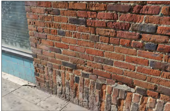
Brick facade, with bricks laid in a common bond pattern. Note the vertical coursing at base (ARG, 2018)
