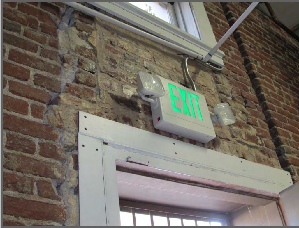
Photo 15: Deterioration of URM wall.
