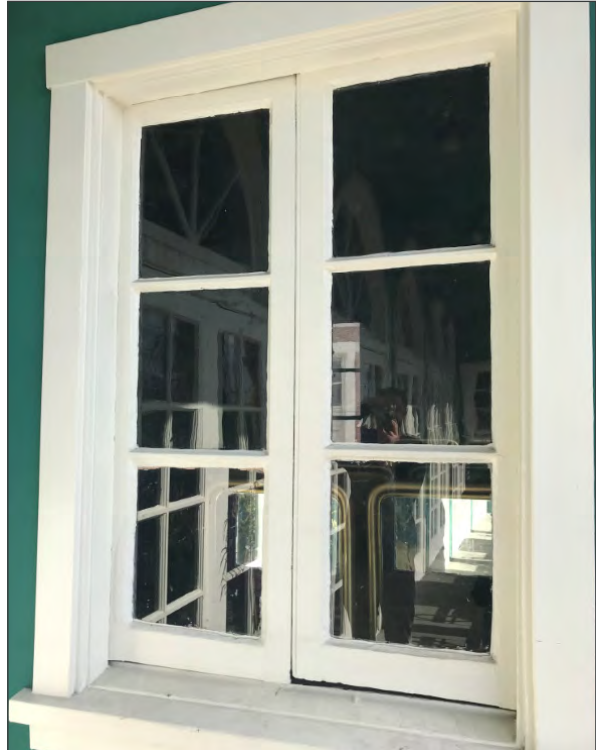
Paired wood casement window at east end of second floor balcony; note misaligned sash (ARG, 2018)
