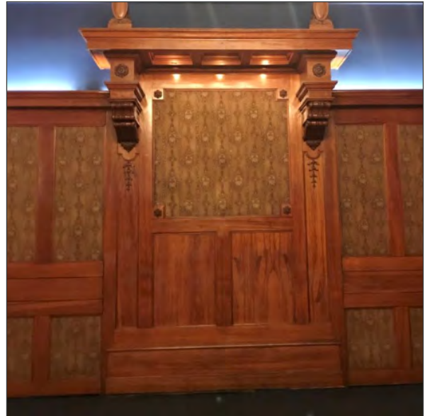
Mural missing at southwest wall (ARG, 2018)
