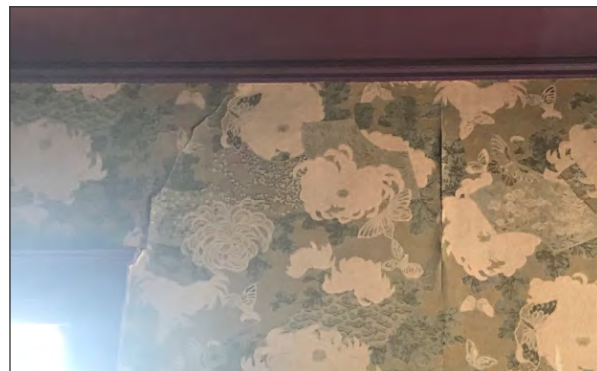
Southeast parlor, damage to wallpaper at northeast wall (ARG, 2018)
