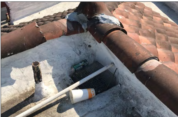
Area drain at east corner of membrane roof. Note trash/debris and loose screen (ARG, 2018)
