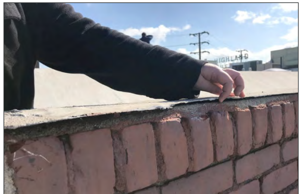
Brick parapet wall. Note loose membrane at top of wall, with no turn down or coping/ flashing. Also note general deterioration of brick masonry (ARG, 2018)
