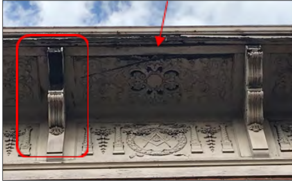
Missing wood bracket and heavily deteriorated/loose wood trim, southeast elevation cornice (ARG, 2018)
