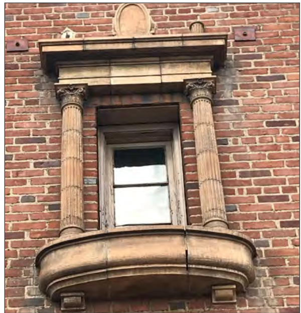
Typical terra cotta window surround at building corner, found on both street elevations (ARG, 2018)
