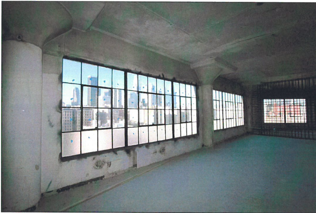
Photo 17: Maxfield Building, 819 S. Santee Street, interior view of typical upper floor open loft, during current adaptive reuse project (Chattel, 2014)
