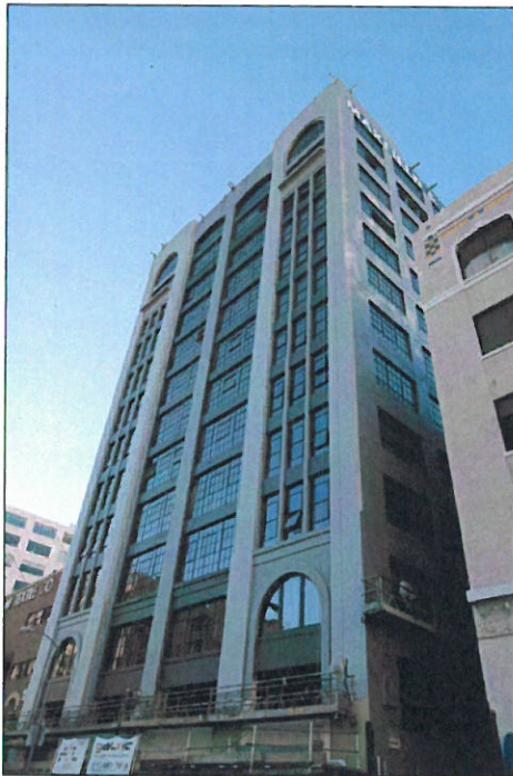
Photo 2: Maxfield Building, 819 S. Santee Street, exterior view southwest of east façade and north elevation, during current adaptive reuse project (Chattel, 2014)
