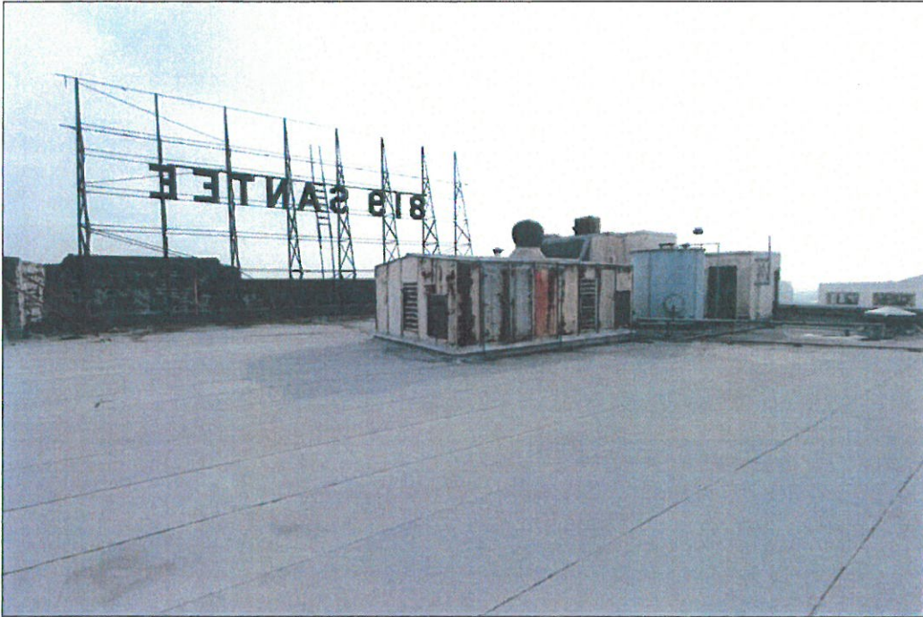
Photo 11: Maxfield Building, 819 S. Santee Street, exterior view southeast of roof (Chattel, Inc., December 4, 2012)
