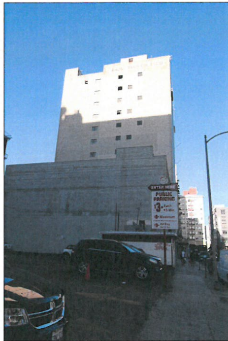
Photo 8: Maxfield Building, 819 S. Santee Street, exterior view north of south elevation, during current adaptive reuse project (Chattel, 2014)
