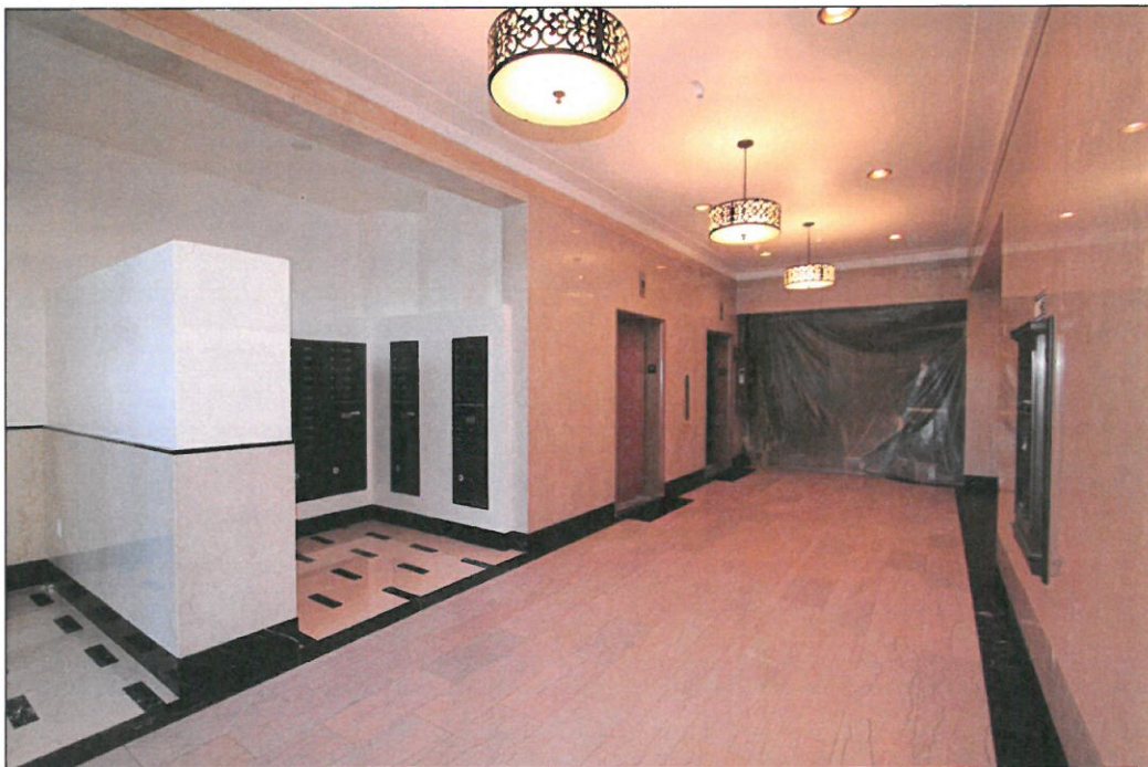
Photo 12: Maxfield Building, 819 S. Santee Street, interior view west of main lobby, during current adaptive reuse project (Chattel, 2014)
