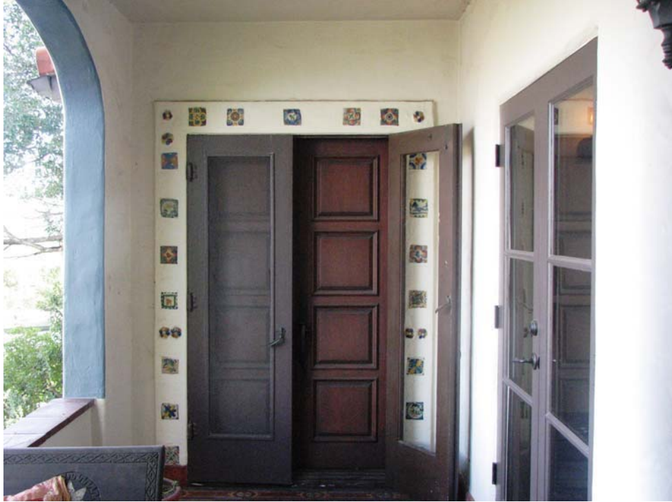
Clarence G. Badger Residence, French doors on second level porch, 7128 Woodrow Wilson Drive, January 28, 2008 (Charles J. Fisher photo)
