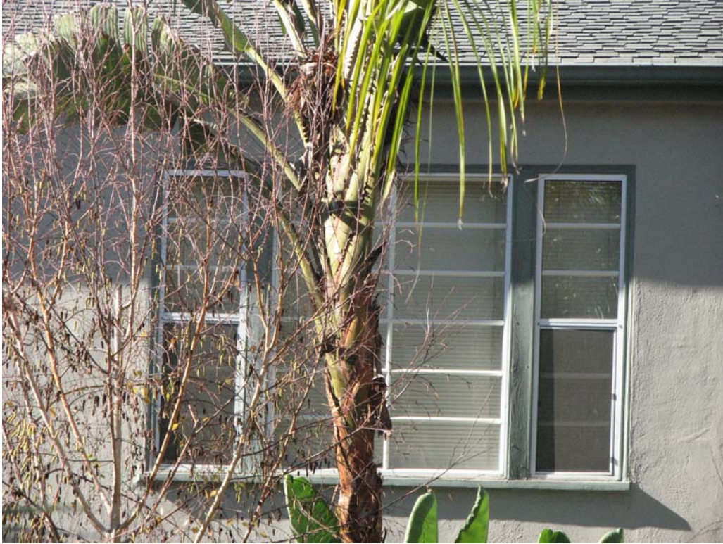
Glen View Garden Apartments, 1801-17 N. New Hampshire Avenue, December 27, 2007 (Charles J. Fisher photo)
