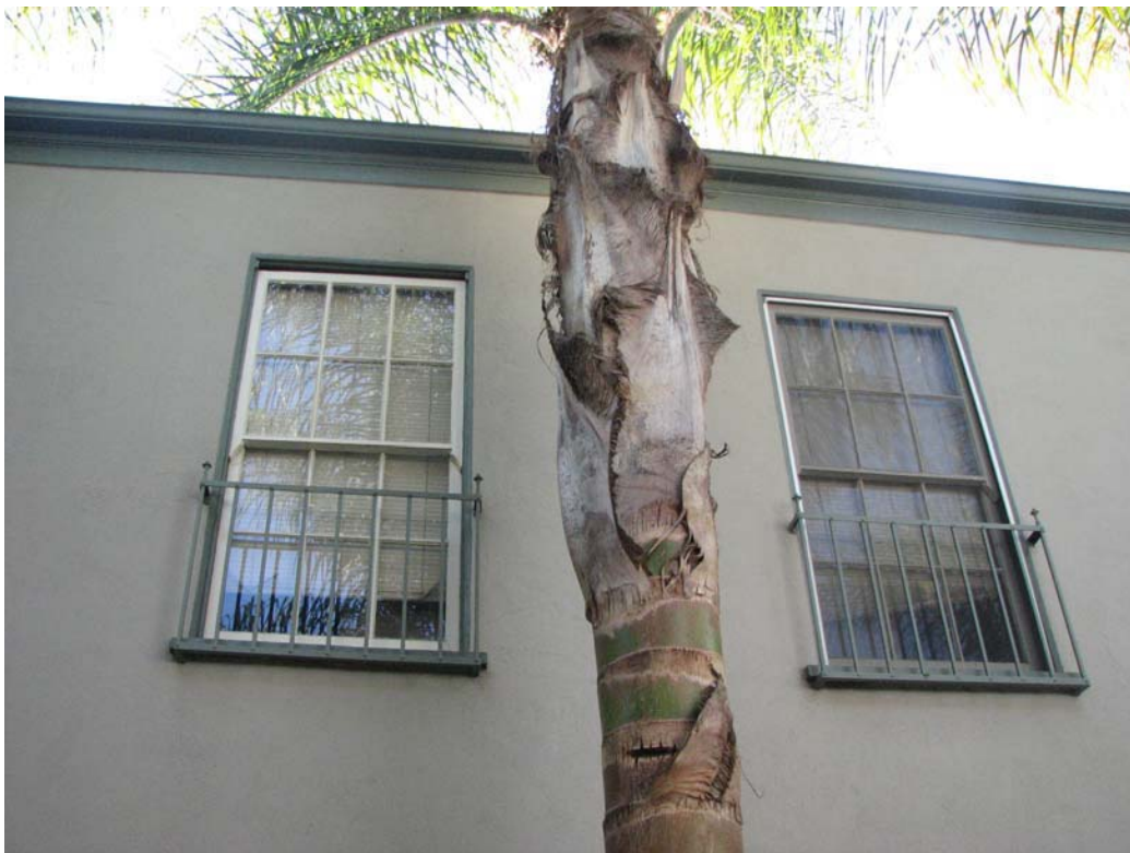
Glen View Garden Apartments, 1801-17 N. New Hampshire Avenue, December 27, 2007 (Charles J. Fisher photo)
