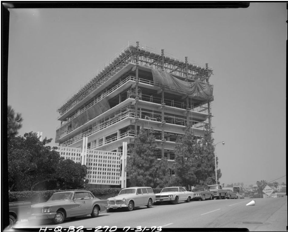
16. Metropolitan Water District Headquarters Campus, High Rise Building under construction, east and north elevations, c. 1972
