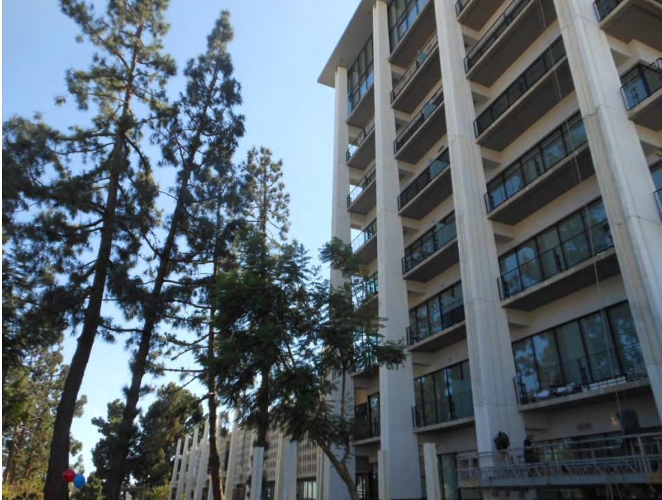
36. Metropolitan Water District Headquarters Campus, Original Building Alpine wing where it meets the High Rise Building, north elevation
