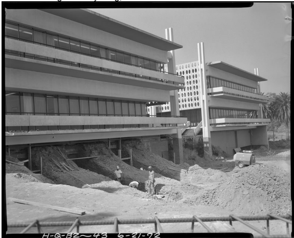
8. Metropolitan Water District Headquarters Campus under construction, Original Building Alpine and Sunset wings, west elevations, c. 1962
