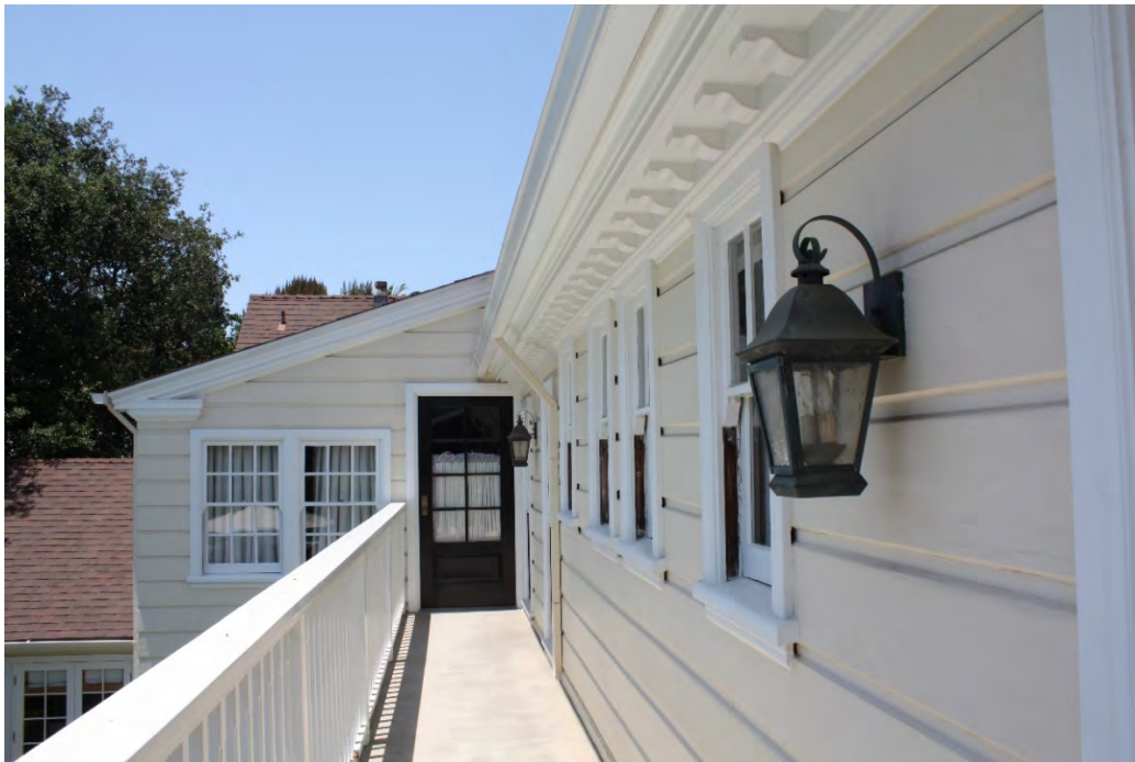
West and south elevations: Upper level balcony/segmented balustrade from south bedroom along south elevation; cornice brackets; two-over-two bathroom windows, view west.
