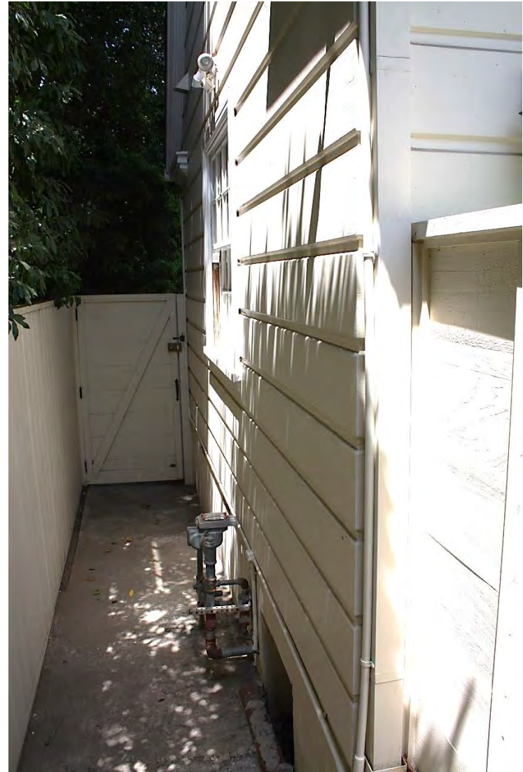
South elevation: South border fence, west gate of same; 6-over-6 double hung window, crawl space vent, southeast corner, view west.
