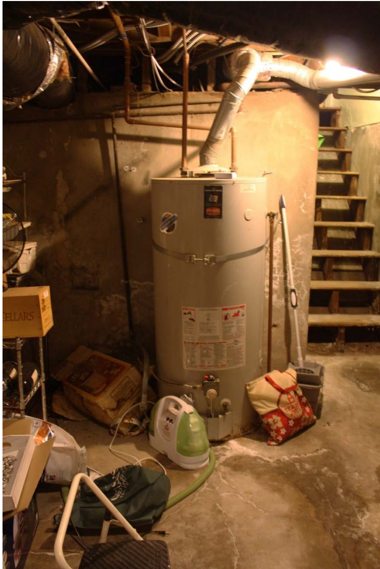
California cellar: Water heater, various plumbing pipes; wood stairs enter cellar.
