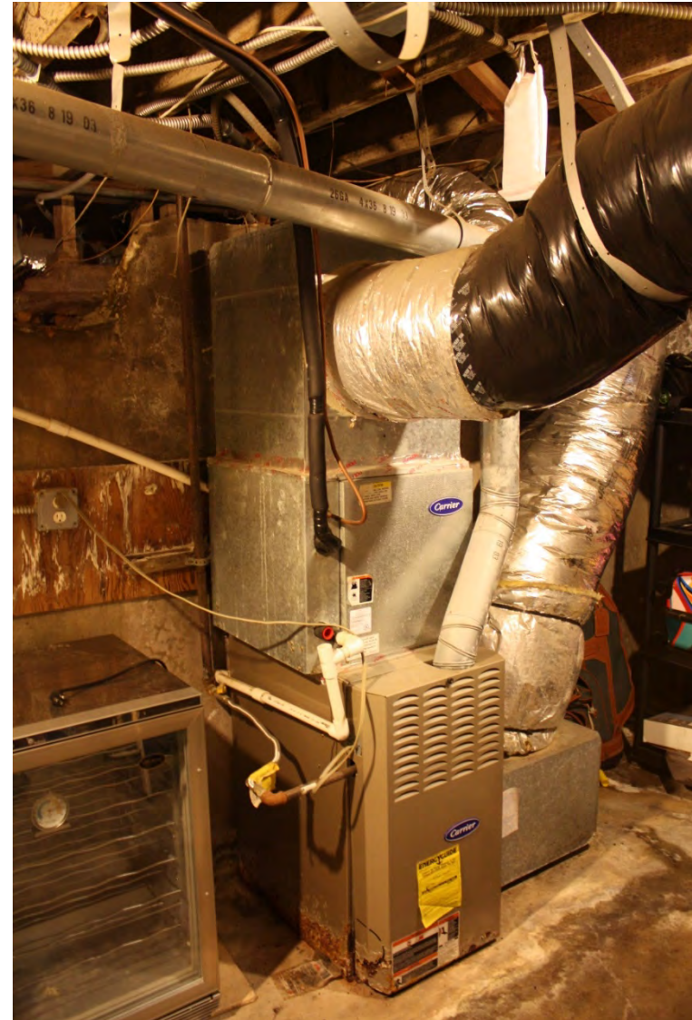
California cellar: Furnace and flues, west.
