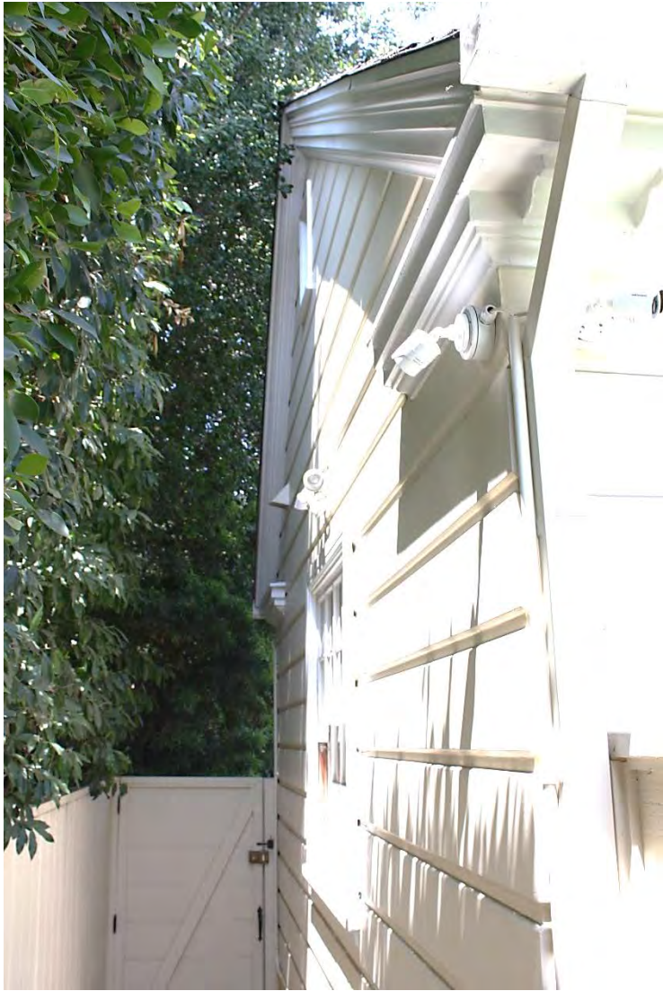
South elevation: South border fence, west gate of same; pedimented gable, vertical vent, 6-over-6 double hung window, southeast corner, view west.
