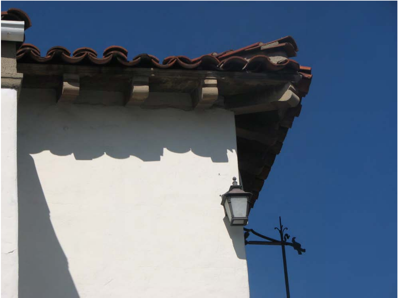
Fred C. Thomson Building, roof tile, light & eaves, 6526-40 Sunset Boulevard, October 24, 2018, (Charles J. Fisher photo)
