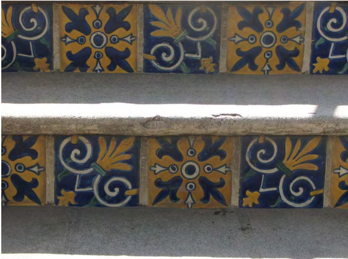
Fred C. Thomson Building, tiles on stair risers, 6526-40 Sunset Boulevard, October 24, 2018, (Charles J. Fisher photo)
