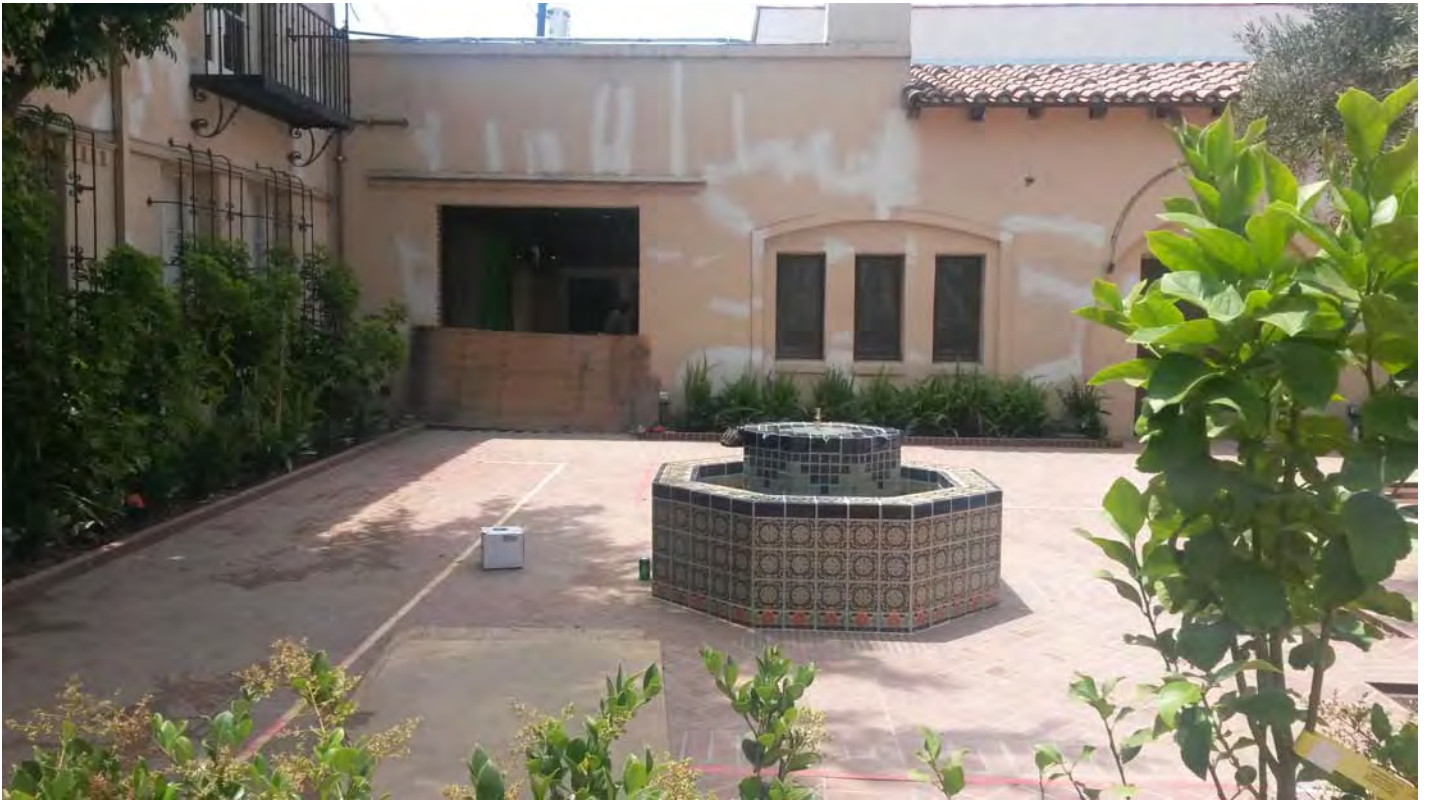
Fred C. Thomson Building, courtyard during work, 6526-40 Sunset Boulevard, May 30, 2017, (Charles J. Fisher photo)
