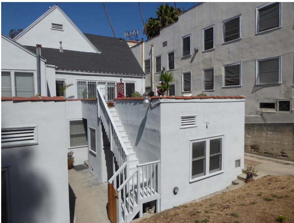
Figure 9: Exterior stair entrance to second floor unit (unit 1922) and terrace above north rear wing (unit 1924) extending into site's slope, east façade facing northwest.
