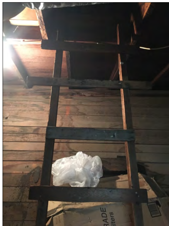
Figure 43: Subject property, interior, 2nd floor, office, view inside one of two access panels to area over sanctuary ceiling, view north (McGee, 2017)
