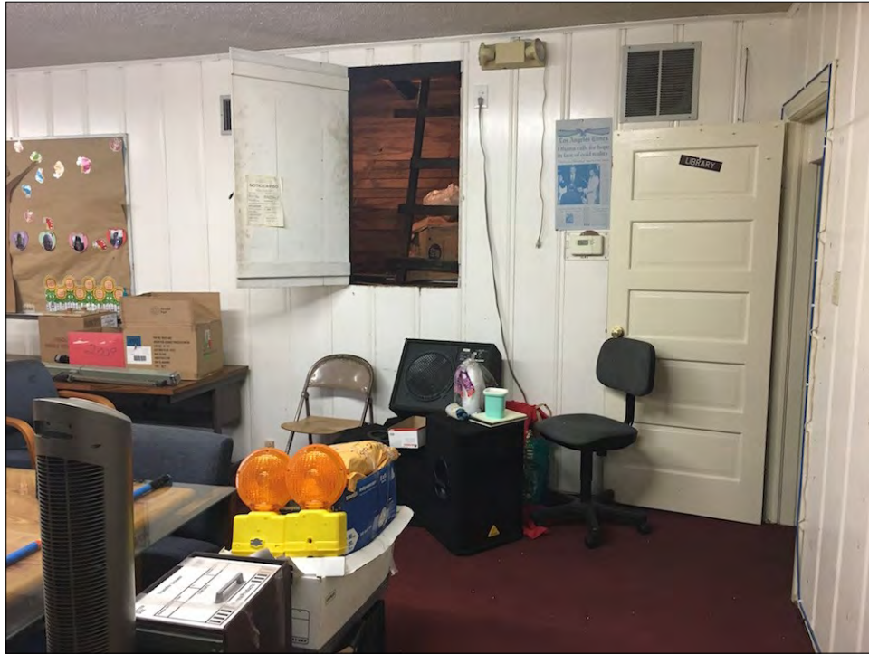
Figure 42: Subject property, interior, 2nd floor, office, north wall showing one of two access panels to area over sanctuary ceiling, view northwest (McGee, 2017)
