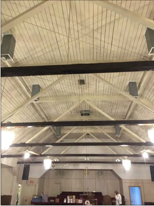
Figure 24: Subject property, interior, 1st floor, sanctuary, detail of ceiling and trusses, view south (McGee, 2017)
