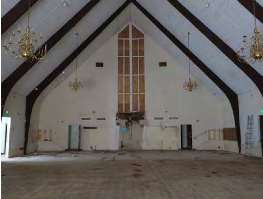
Sanctuary main room, view north (ARG, 2018). The glazing in the north clerestory has been removed.
