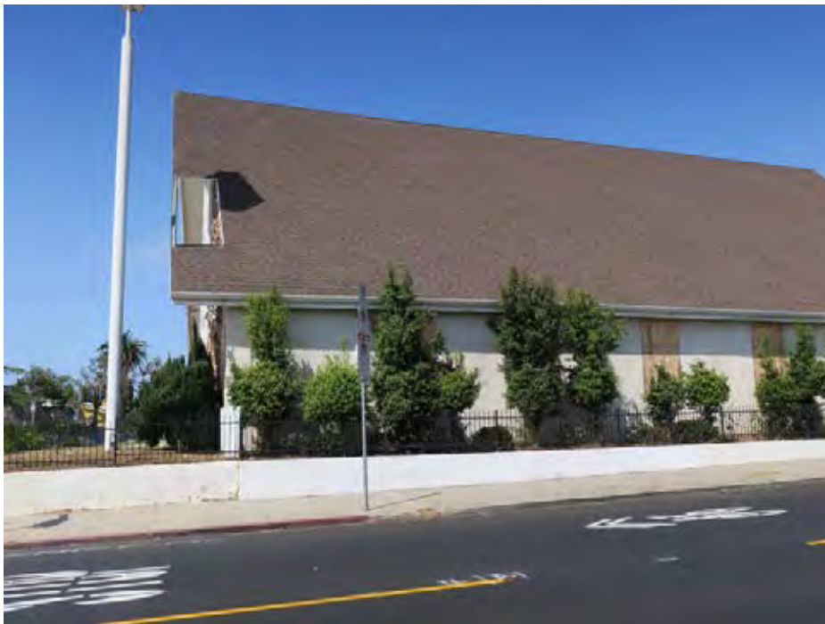
View west illustrating the rectangular roof opening where a stylized metal cross sculpture historically stood adjacent to the primary façade (ARG, 2018).
