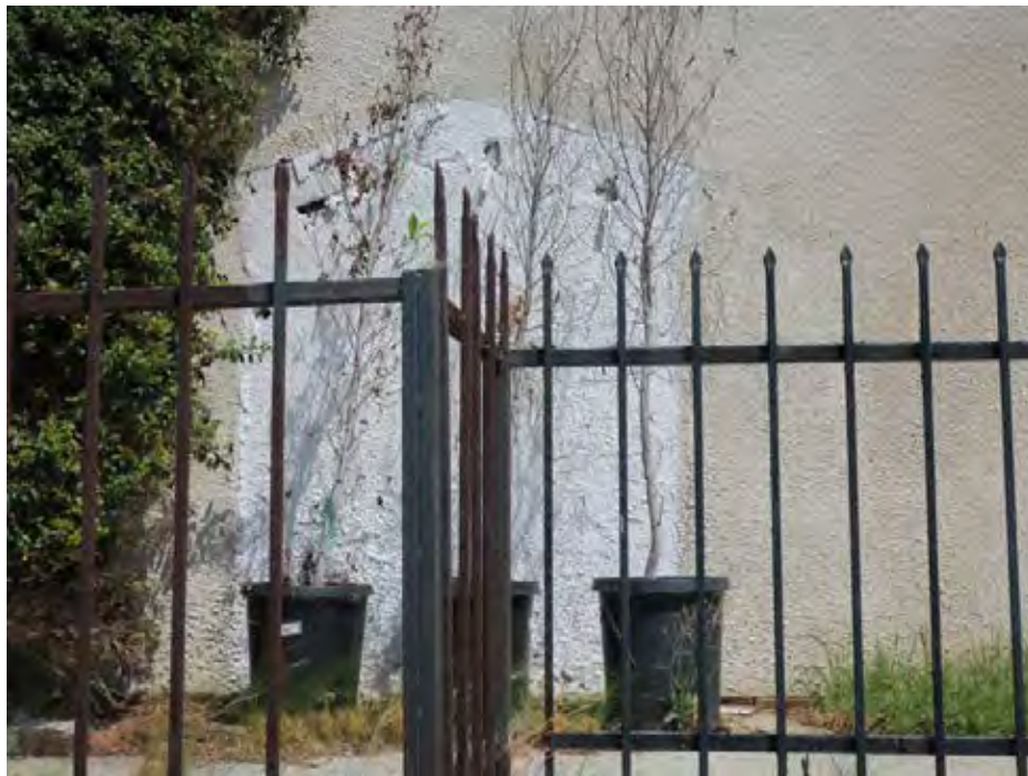
Detail view at the western south façade of the education wing (ARG, 2018). The original church reader board has been removed and leaves a ghost in the stucco.
