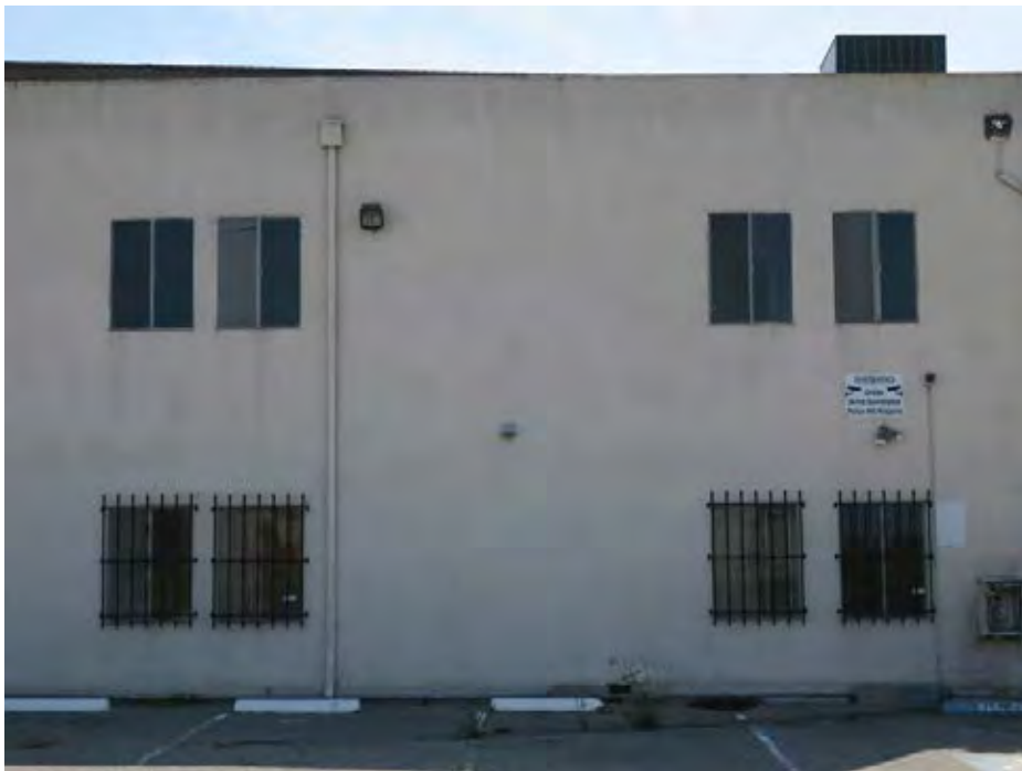
View of the fenestration at the southern west façade featuring aluminum slider windows (ARG, 2018).
