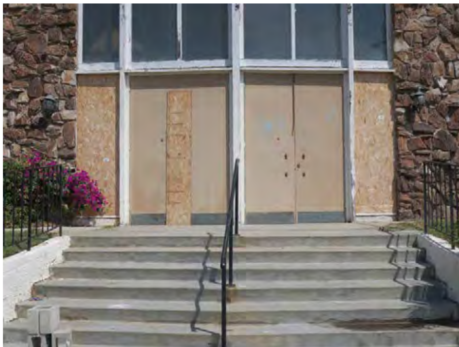
View north at the sanctuary main entrance (ARG, 2018). Doors have been stripped and sidelights have been removed.
