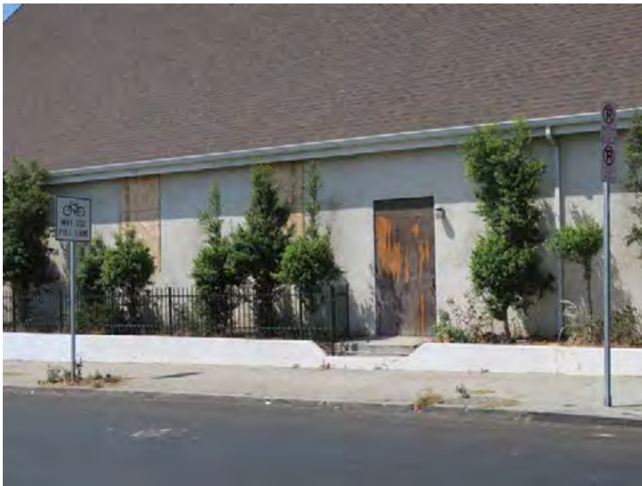
View southwest at a secondary entrance to the sanctuary (ARG, 2018). The door is warped and the windows to the south have been removed.
