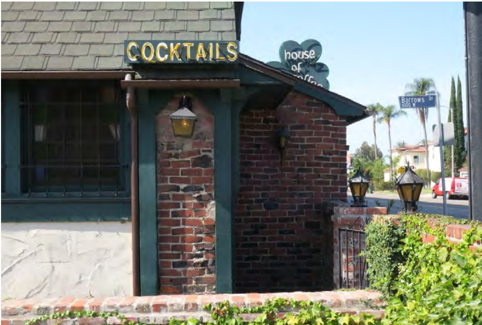
Primary (north) elevation, detail of clinker brick and textured stucco, view south (ARG, 2018).
