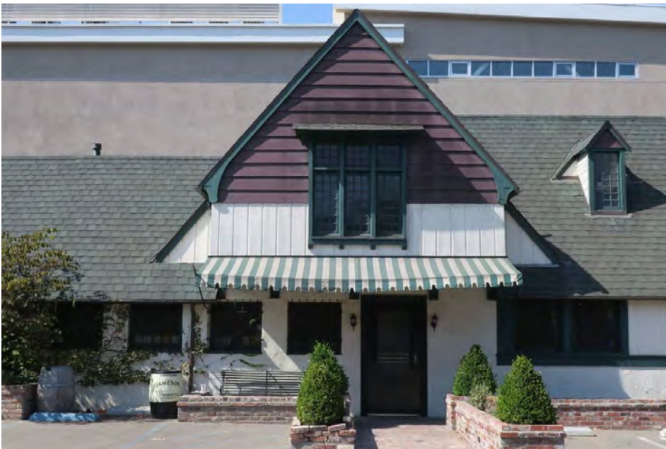
Primary (north) elevation, detail of jettied gable and entrance, view south (ARG, 2018).
