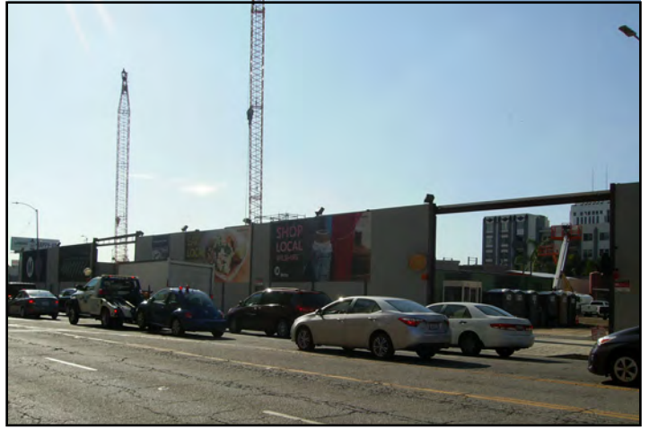
View 7: From the east side of La Brea Avenue, looking southwest at the construction of a Metro Purple Line station.
