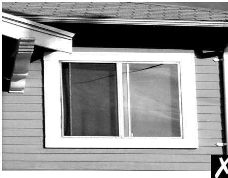
These sliding aluminum replacement windows are inappropriate.
