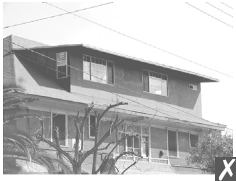
Inappropriate rooftop addition located on a street-facing facade with incompatible windows
