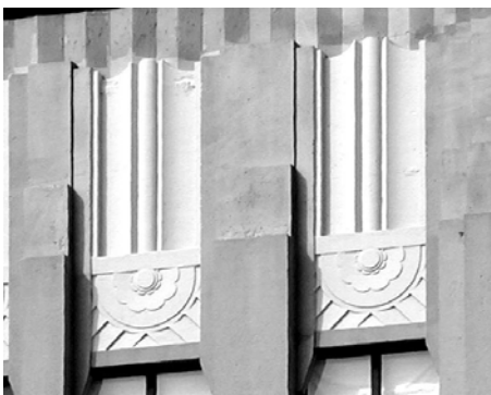
Concrete detail like this should not be cleaned with aggressive abrasive methods, or the detail may be lost.
