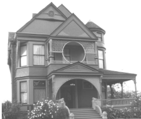
Roof and eave details, such as rafter tails, vents, corbels, built in gutters and other architectural features shall be preserved.
