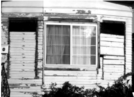
Filling in historic window openings is inappropriate.
