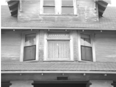
Generally, historic windows should not be replaced unless they cannot be repaired or rebuilt.
