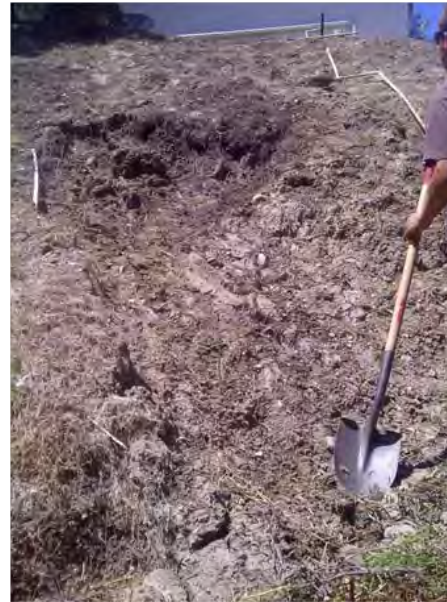
Difficult Repair of Pop Out
