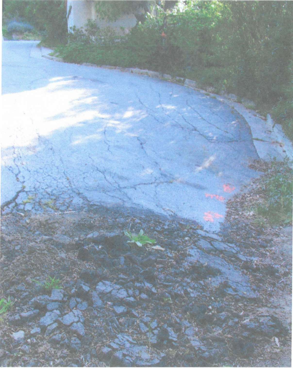
D-2. Upwelling and percolation of water has repeatedly and significantly damaged San Andreas Avenue.
