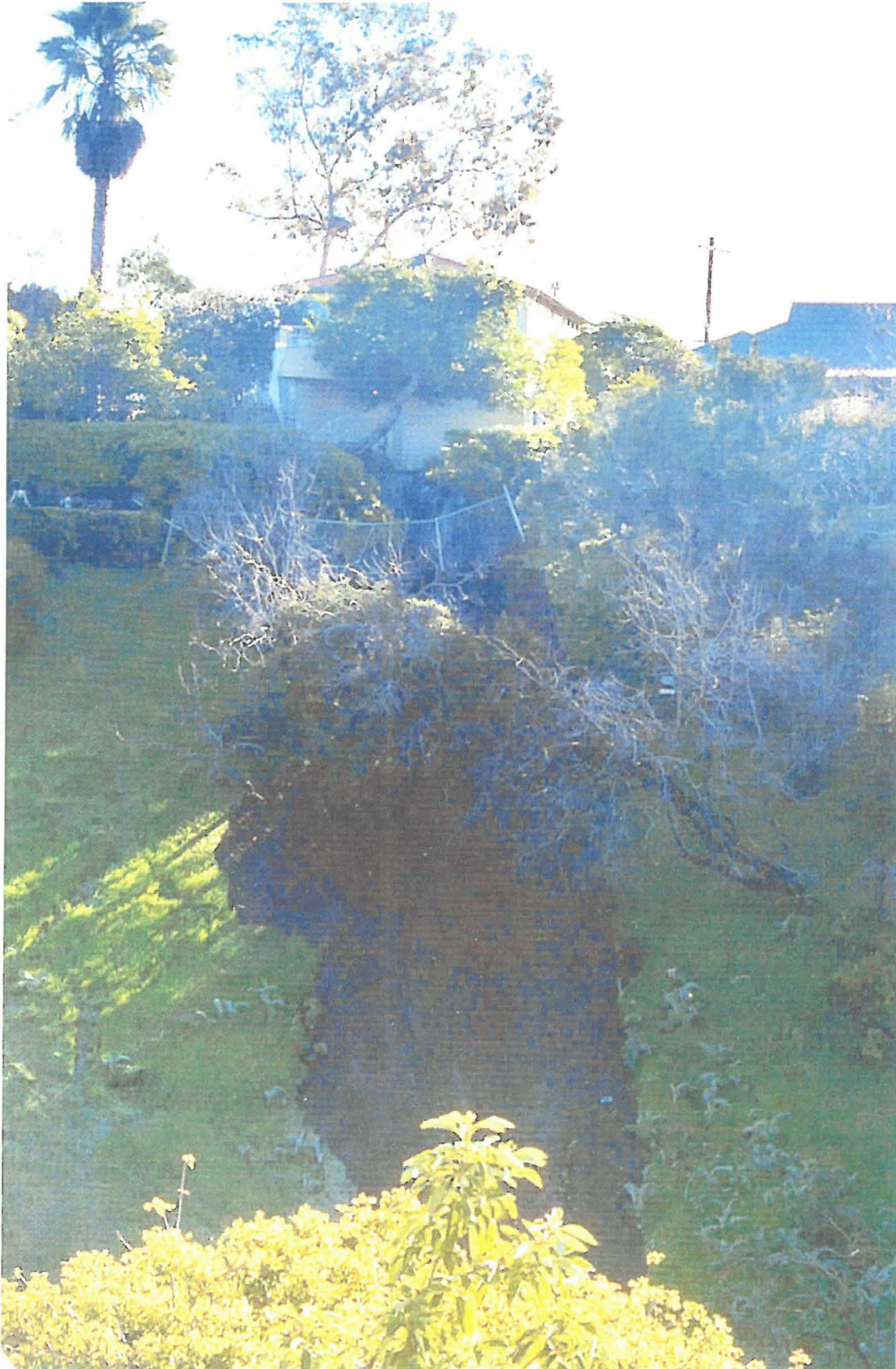
E-1. Landslide Winter 2005-2006. This landslide began in Red Hawk Canyon and destroyed the foundation of a deck at 4267 San Rafael Avenue.
