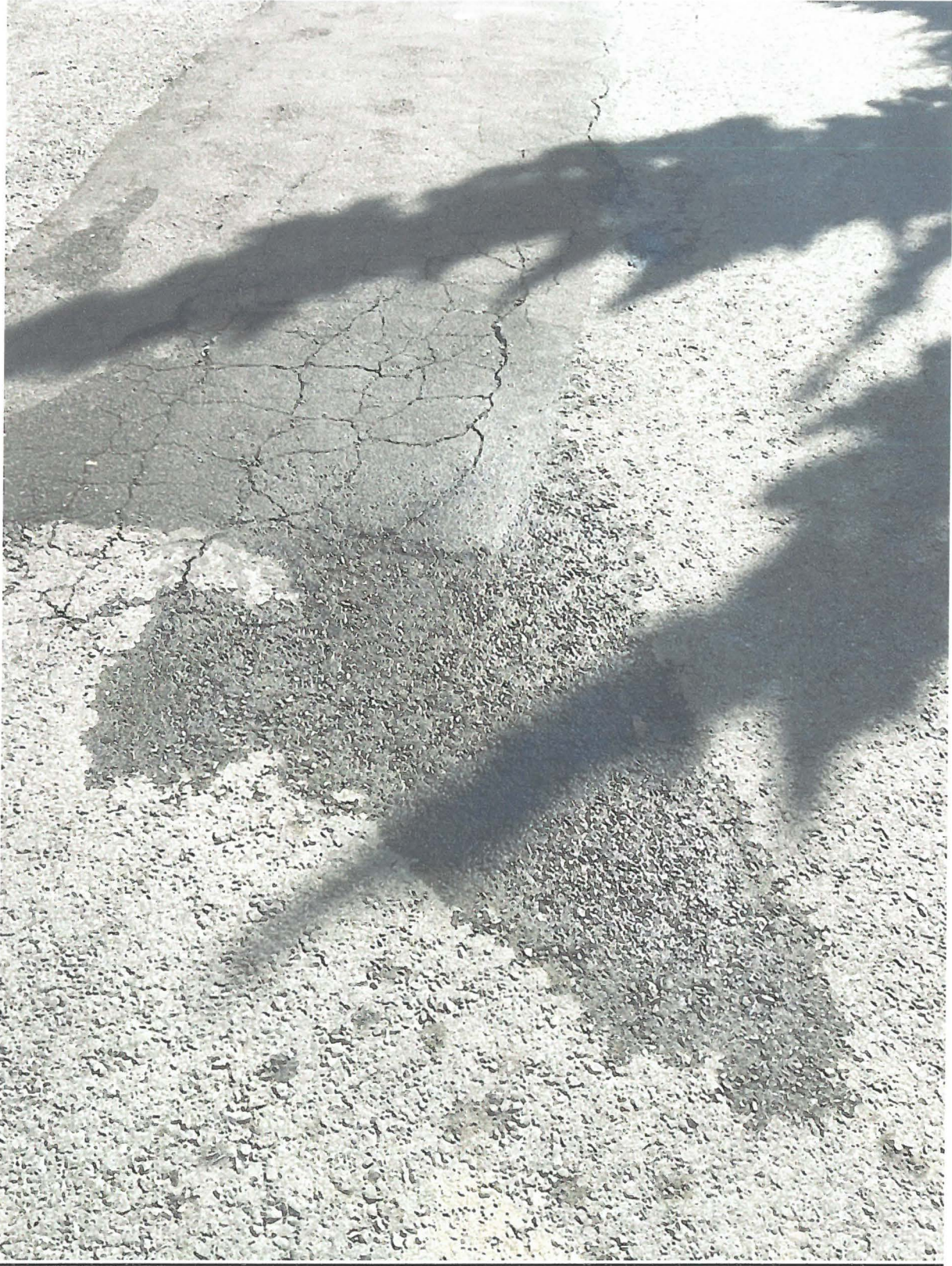
D-1. Upwelling and percolation of water has significantly and repeatedly damaged Cynthia Avenue.
