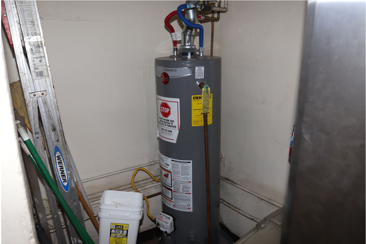
Changed plumbing and new water heater
