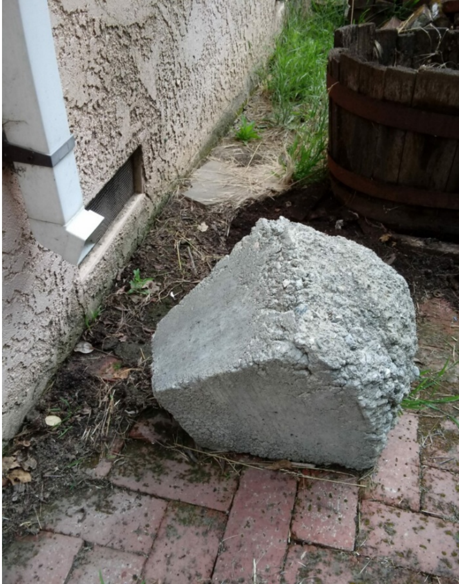
Photo 5: Landslide at 805 Cynthia Ave. Concrete foundation
