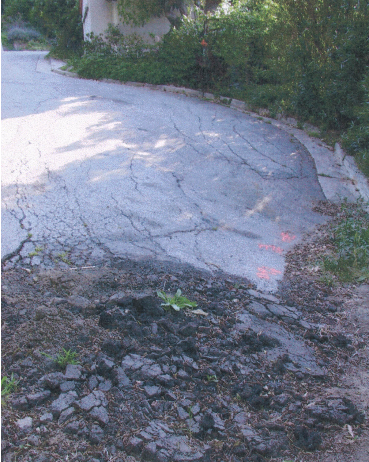
Photo 3: Upwelling on San Andreas Ave. (north of RHC) due to subsurface water flow
