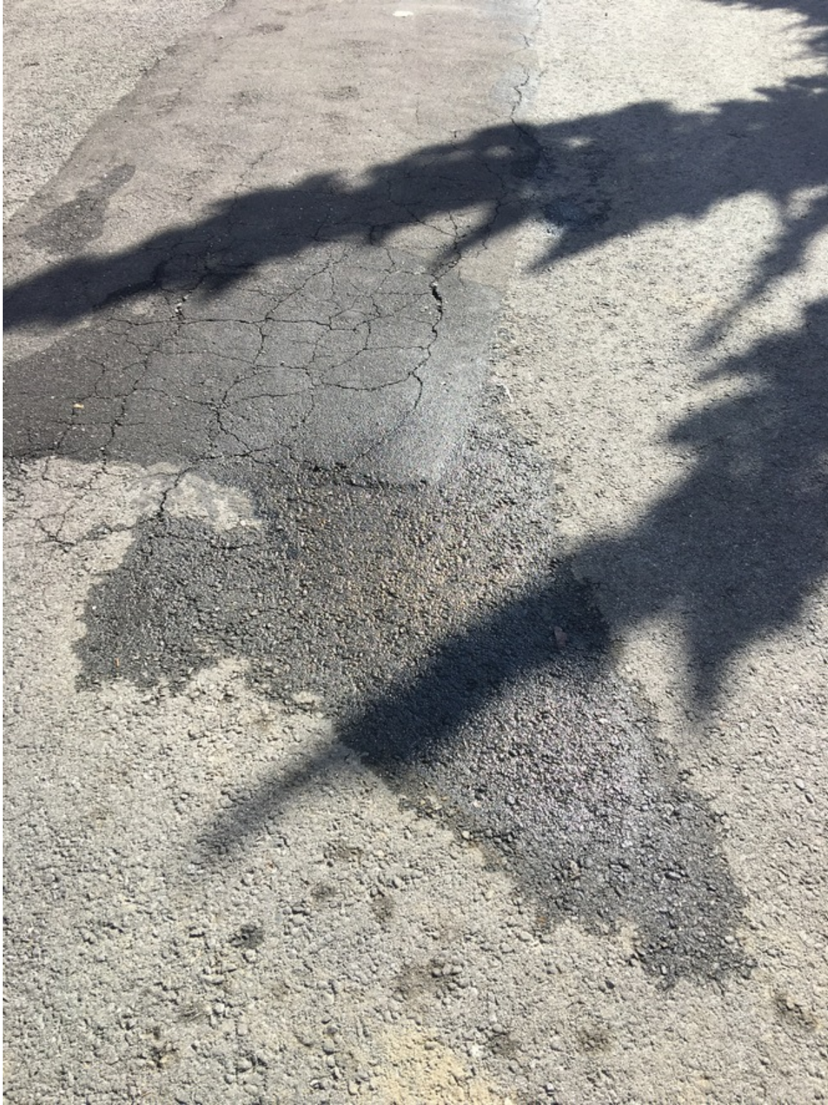
Photo 2: Upwelling on Cynthia Ave. (south of RHC) due to subsurface water flow
