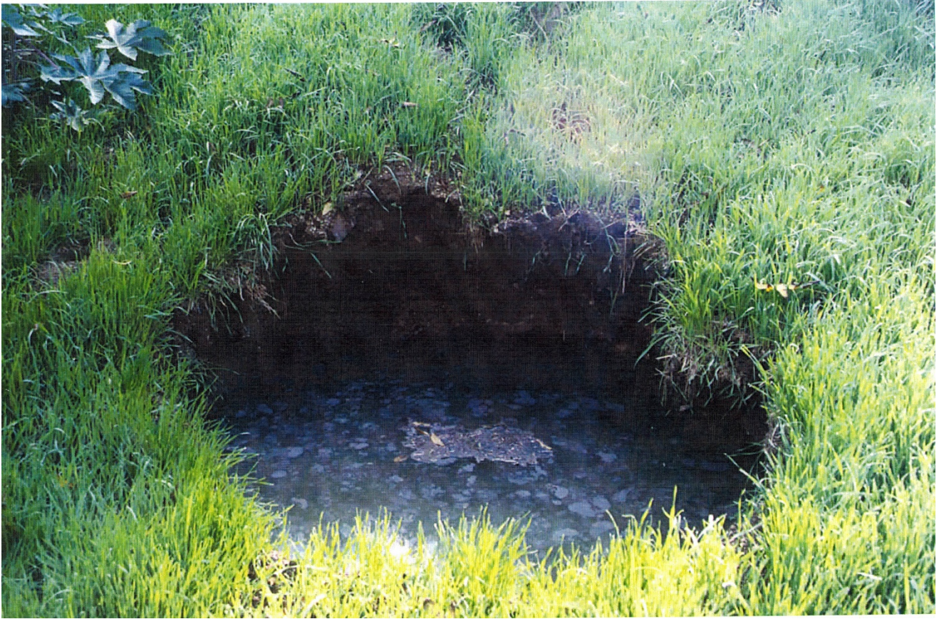
Photo 7: Sinkhole in RHC
