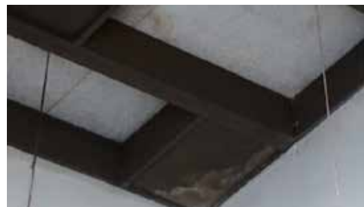
Figure 3 Water Damage. Photo: Peyton Hall
