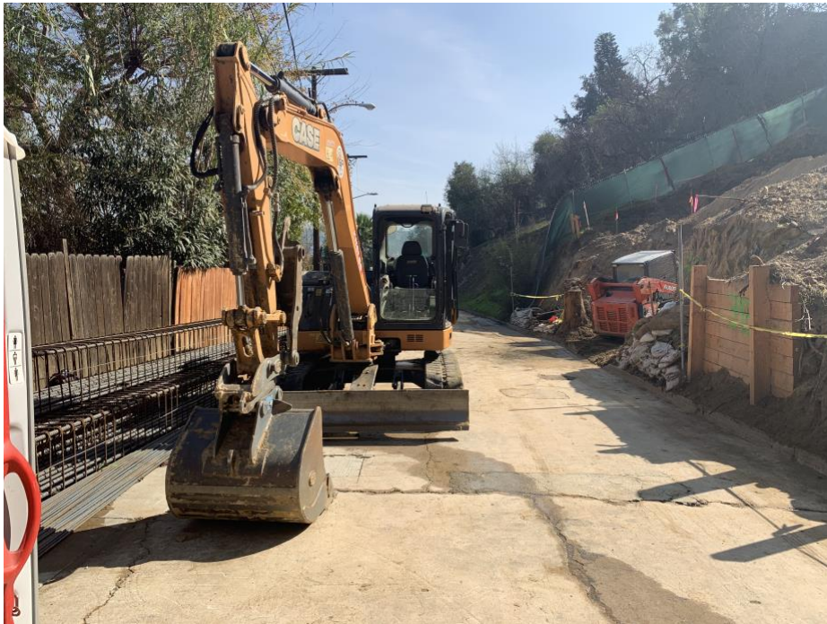
Construction debris, materials and equipment stored on roadway, narrowing it to 9 feet and blocking access for any emergency vehicle or even regular traffic
