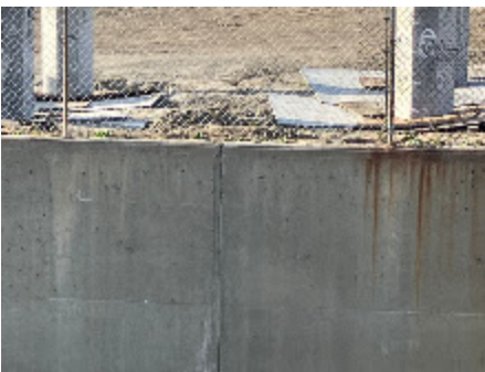
IMG_0827 vertical offset at separation_north wall.jpg 985K
