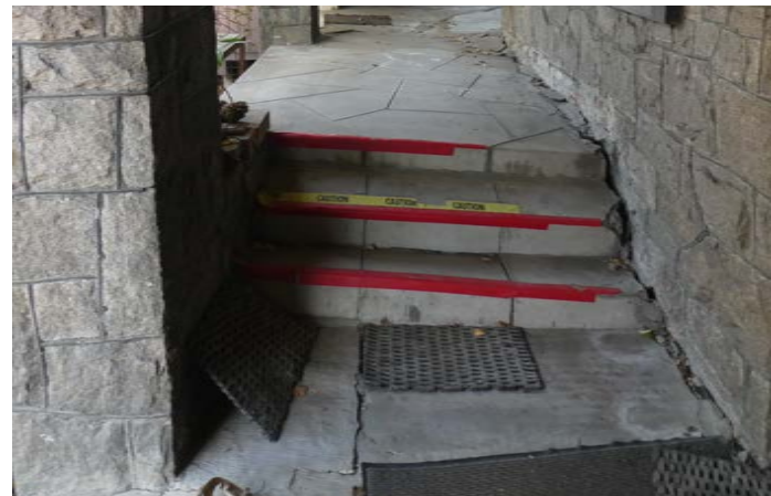
Figure 7: Differential settlement at porch on west elevation (GPA, 2019)
