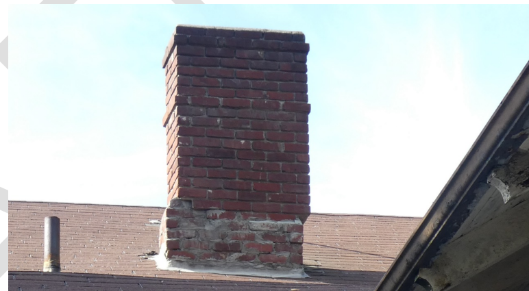
Figure 9: Tilting brick chimney on east side of roof (GPA, 2019)
