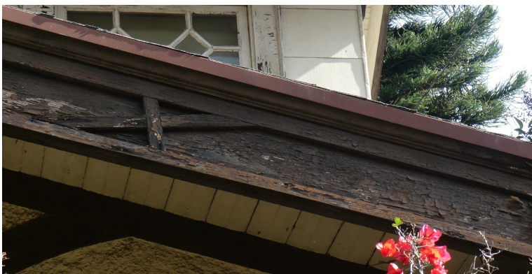
Figure 8: Porte-cochere on west elevation, wood deterioration at ornamental rake (GPA, 2019)
