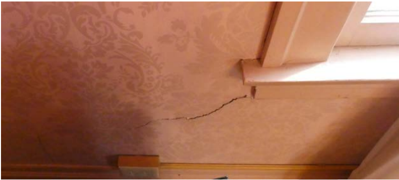
Figure 10: Southeast bedroom on the second floor, stress crack in the plaster on the east wall (GPA, 2019)
