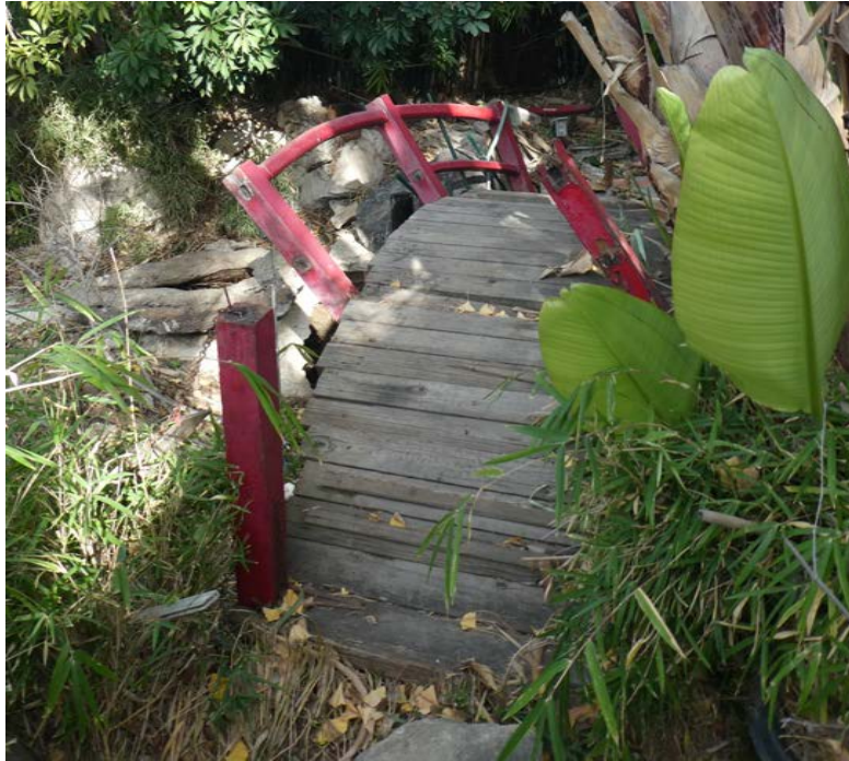
Figure 6: Foot bridges in the Japanese garden are in poor condition (GPA, 2019)
