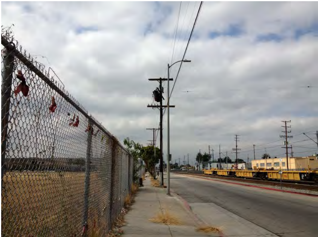
Photo 14 - Pole-mounted transformer, west of the Property
