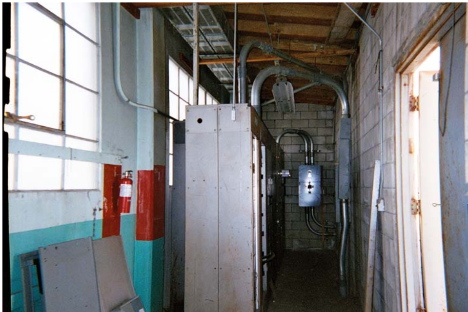
Photograph 14: Inside the Teledyne Controls transformer station.
