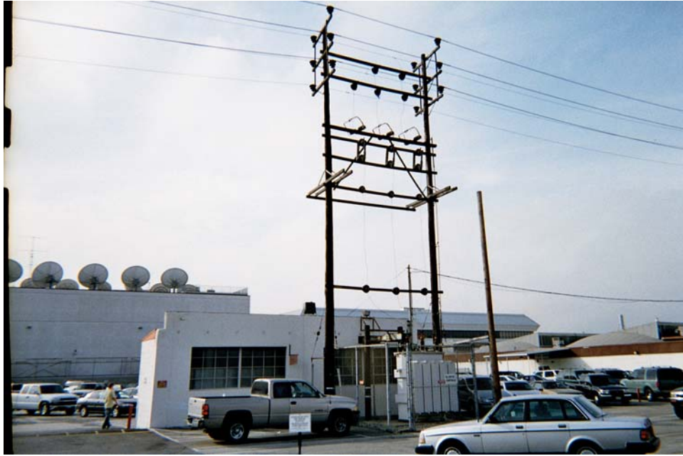
Photograph 13: Teledyne Controls transformer station.
