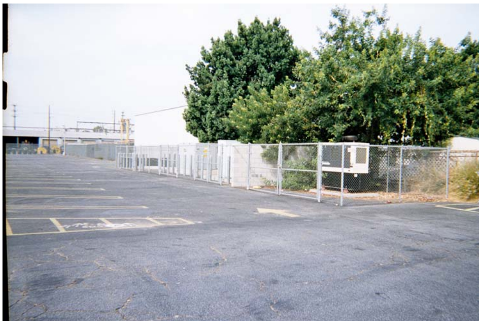
Photograph 8: Transformers to the south of building at 1901 S. Bundy Drive.
