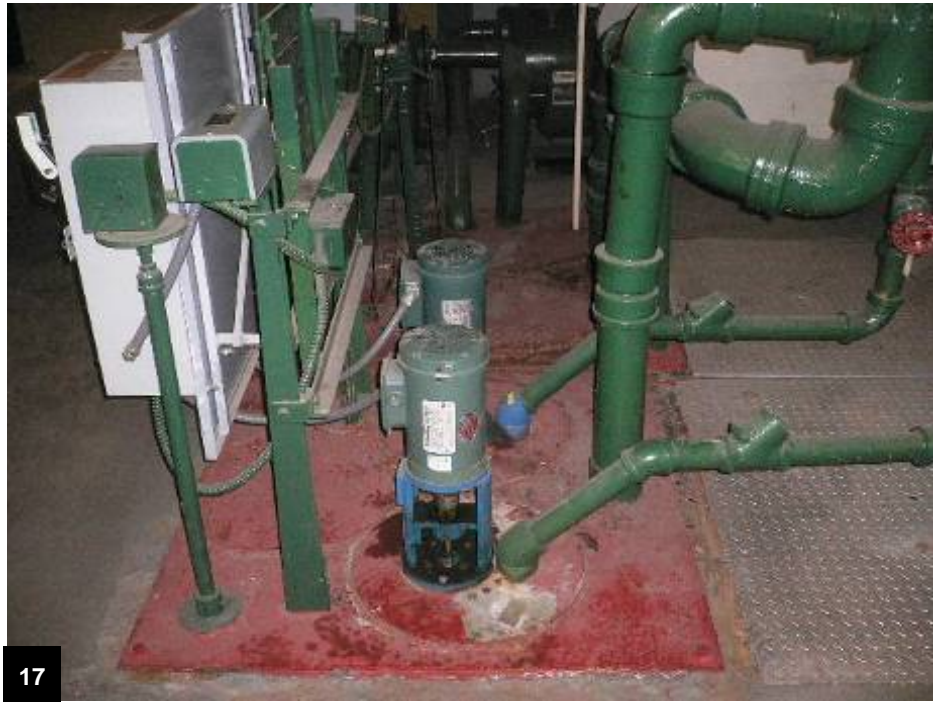
Sumps and interceptor
