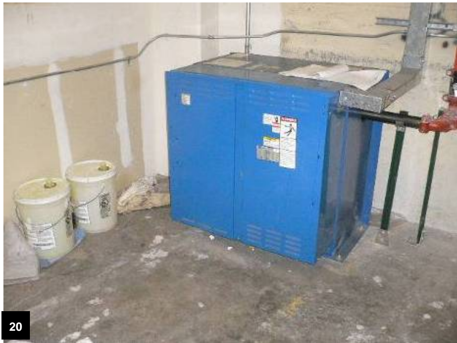
Hydraulic elevator machinery for spa
