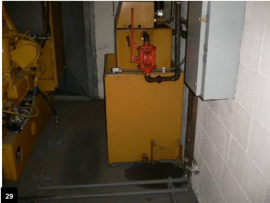
Day tank for emergency generator #2
