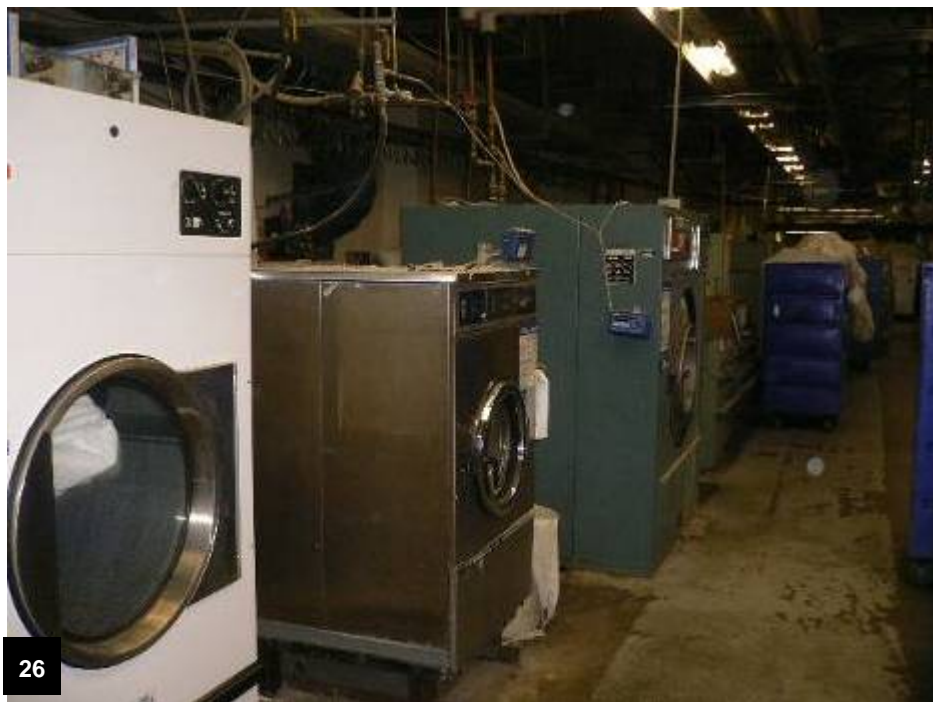
Washers in laundry area
