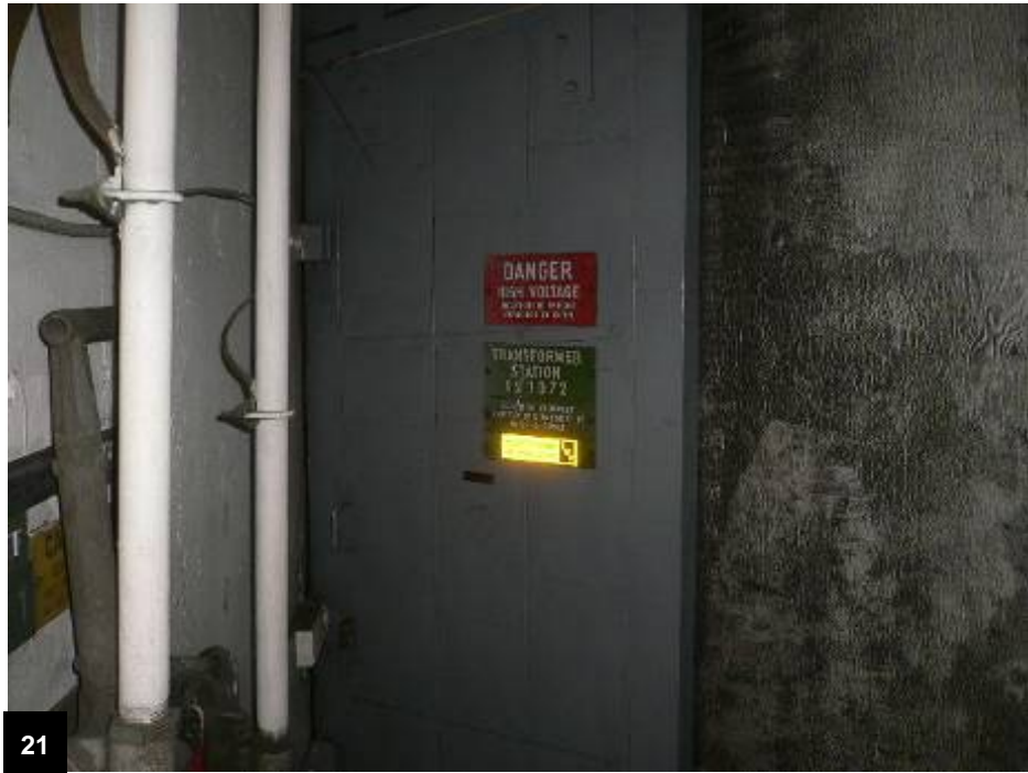
DWP transformer room
