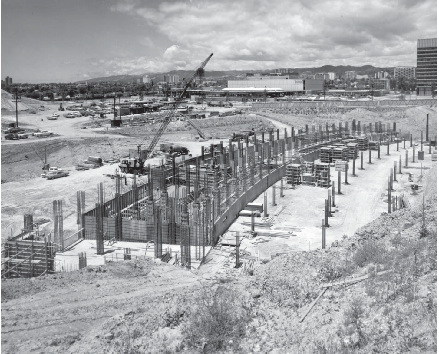
View of Century Plaza Hotel foundation, crescent footprint, c. 1965. (Source: Courtesy Westin Hotels & Resorts, Image No. 656b291f69_20.)
