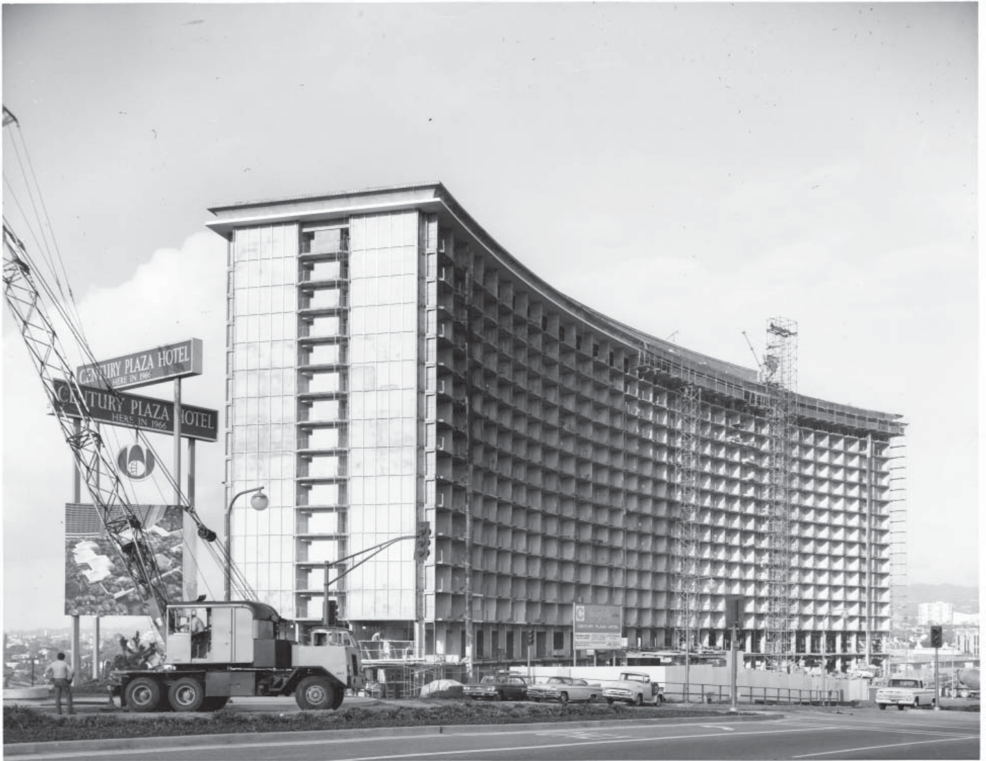
Exterior view of hotel under construction, dated 19 November 1965. (Source: Courtesy Westin Hotels & Resorts, Image No. 656b291f69_47.)
