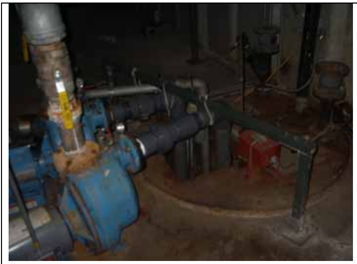
23. View of sump pump of the de-watering system in subterranean parking garage P4.
