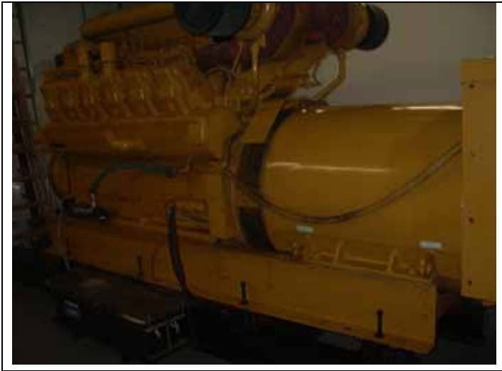
19. View of an emergency generator on the ground floor of the office building.
