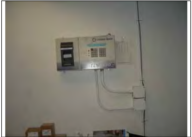
20. View of leak detection monitor for the diesel UST at the ground floor of the office building.
