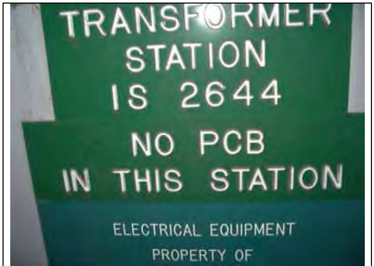
22. View of LADWP transformer room in subterranean parking garage P2.
