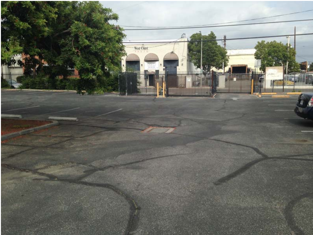
View of the parking area & surface drain north of the subject property building looking E 1116 N McCadden Place & 6725 Santa Monica Blvd, Los Angeles
