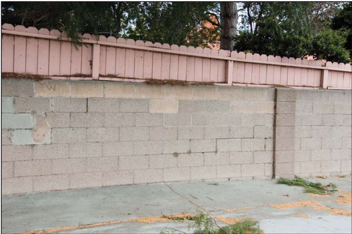
Views of the masonry wall that separates homes along Tarrasa Drive from Western Avenue.
